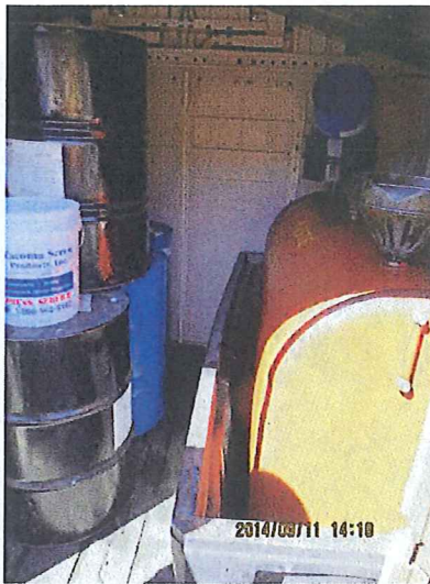
#7. DESCRIPTION: Waste Oil Shed, showing containment for waste oil tank. No berm or raised lip on floor of shed to prevent potentially spilled oil from reaching outdoor area.
