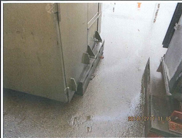
15 DESCRIPTION: CLOSE UP OF SHEEN FROM TRANSFORMERS IN PHOTO 13. FLOWING WESTWARD TOWARD CATCH BASIN VISIBLE IN PHOTO 12.
