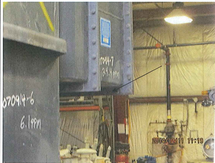
11 DESCRIPTION: CLOSE UP OF OLD TRANSFORMER FROM PHOTO 10 SHOWING PCB CONTENT OF COMPONENTS (6.1 PPM, 24.4 PPM)
