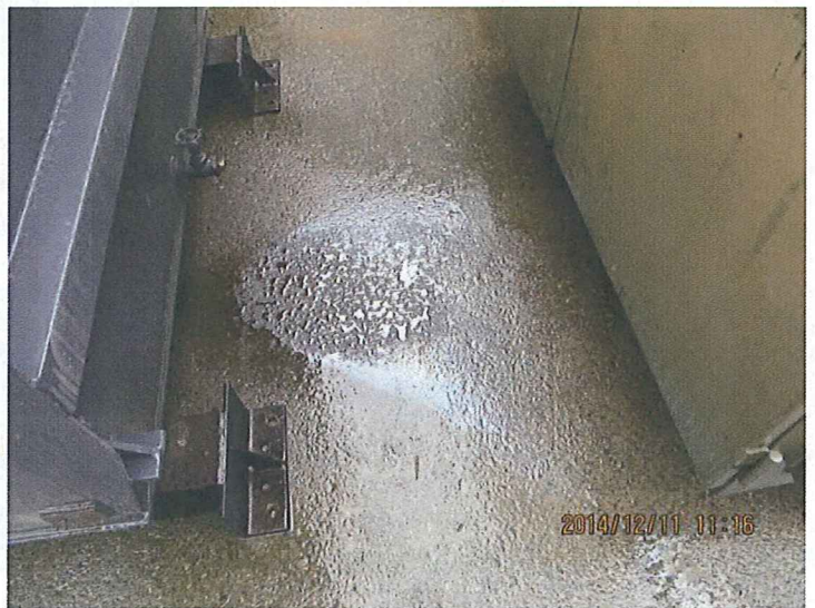
14 DESCRIPTION: CLOSE UP OF OIL STAINS AND SHEEN IN TRANSFORMER STORAGE AREA (SAME AS IN PHOTO 13).
