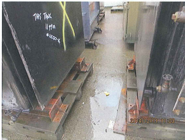
13 DESCRIPTION: NORTH SIDE OF PCB BUILDING, LOOKING SOUTH BETWEEN STORED TRANSFORMERS (SAME AS IN PHOTO 12). SHEEN AND OIL STAINS.
