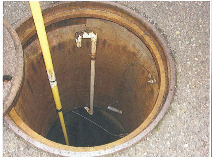
16 DESCRIPTION: SOLIDS MATERIAL ON TOP OF STANDPIPE INSIDE OIL WATER SEPARATOR MANHOLE (DRAINAGE AREA F)
