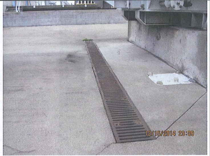
08 DESCRIPTION: TRENCH DRAIN INSIDE LARGE TRANSFORMER CONTAINMENT PAD
