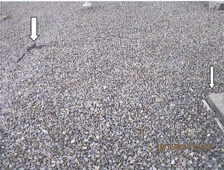
05 DESCRIPTION: ARROWS SHOW EDGES OF IMPERMEABLE LINER TO PREVENT INFILTRATION OF SPILLS FROM ADJACENT OIL CIRCUIT BREAKER
