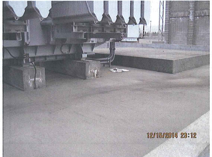
06 DESCRIPTION: LARGE TRANSFORMER CONTAINMENT PAD (CONCRETE CURBED), WEATHERED ABSORBENT PAD UNDER VALVE, PAVEMENT STAINING
