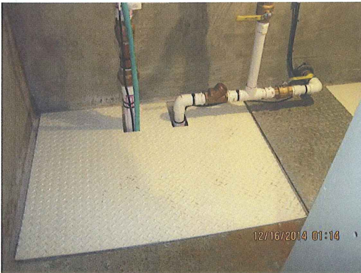
11 DESCRIPTION: : CONTROL HOUSE BASEMENT SUMP PUMP TO STORMWATER SYSTEM (CLOSED)
