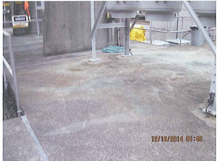
04 DESCRIPTION: PAVEMENT STAINING BENEATH TRANSFORMERS
