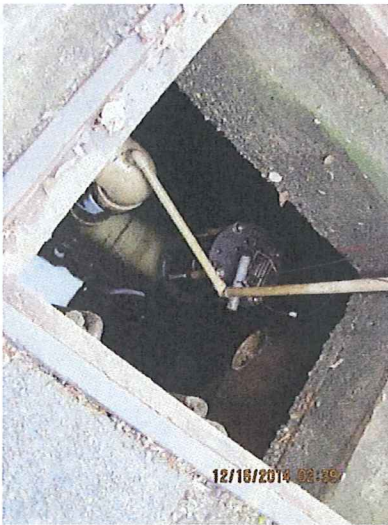
15 DESCRIPTION: CATCH BASIN EQUIPPED WITH AN AUTOMATIC SHUTOFF VALVE (FLOAT SWITCH OPERATED)
