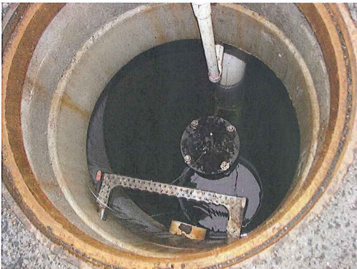
17 DESCRIPTION: SOLIDS MATERIAL ON TOP OF SHUTOFF VALVE INSIDE A MANHOLE IN DRAINAGE AREA F
