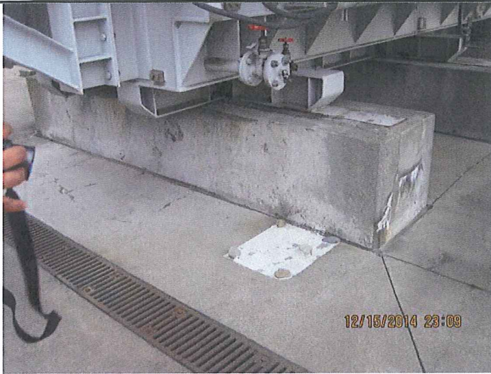
07 DESCRIPTION: WEATHERED ABSORBENT PAD UNDER VALVE IN PROXIMITY TO TRENCH DRAIN
