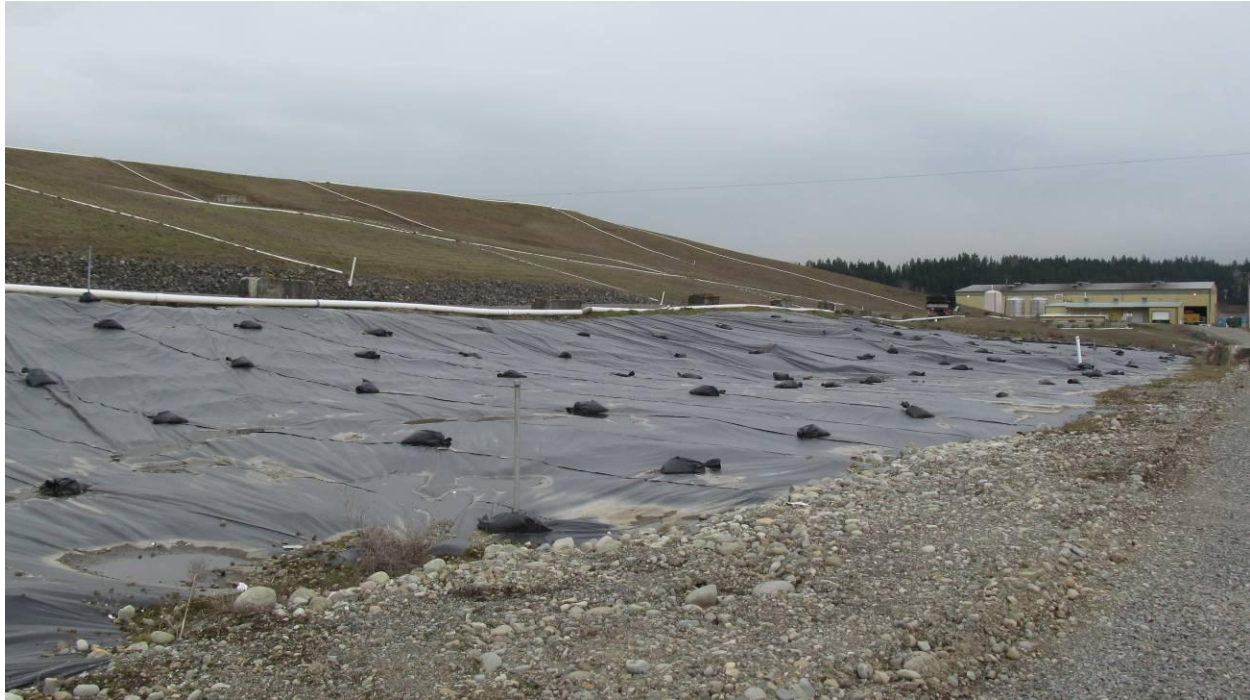
Photo 1: Landfill Sink Hole Area – from the southwest
