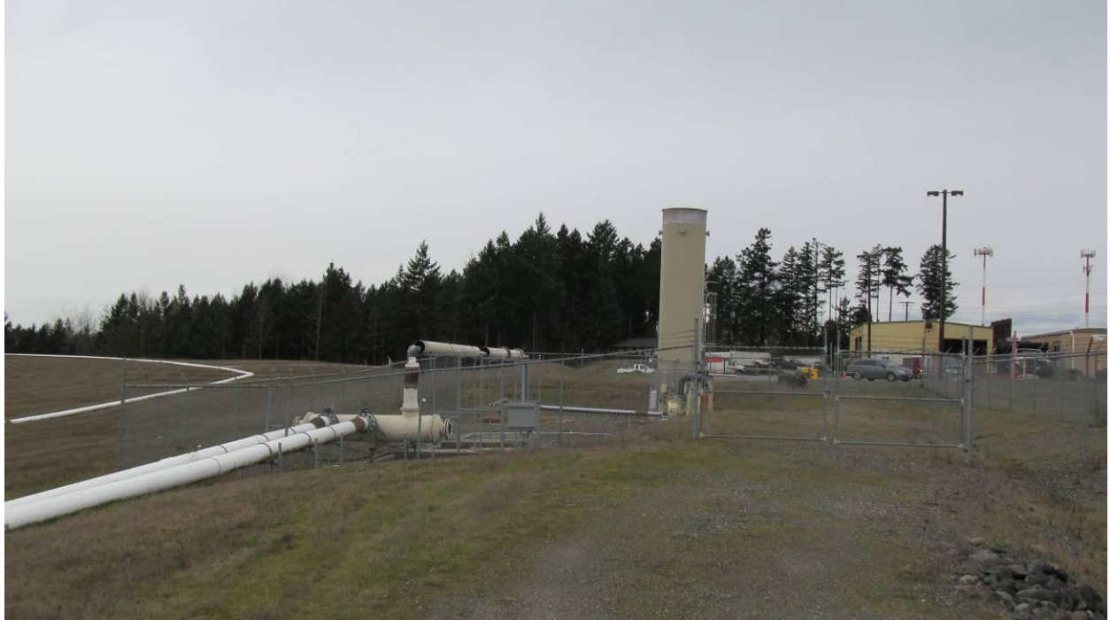
Photo 3: Gas Collection Flare - from the east
