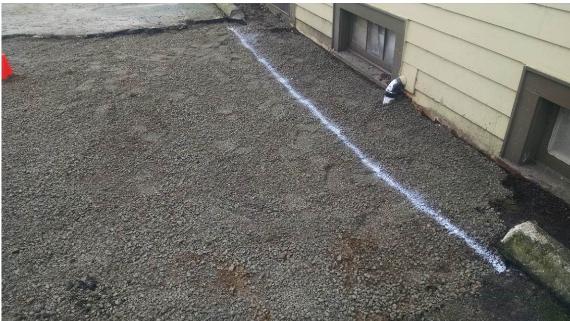
Photograph 9 – Surfacial backfill brought to grade and prepared for asphalt surfacing. 4-inch well location marked with cone. Well monument subsequently replaced prior to asphalt paving.
