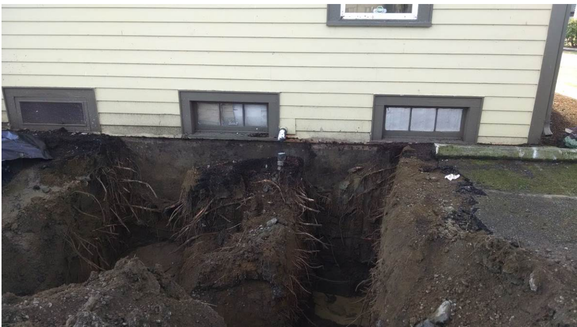
Photograph 5 – East and west 'cells' after soil removal, with remnant center cell in place, January 13, 2015.
