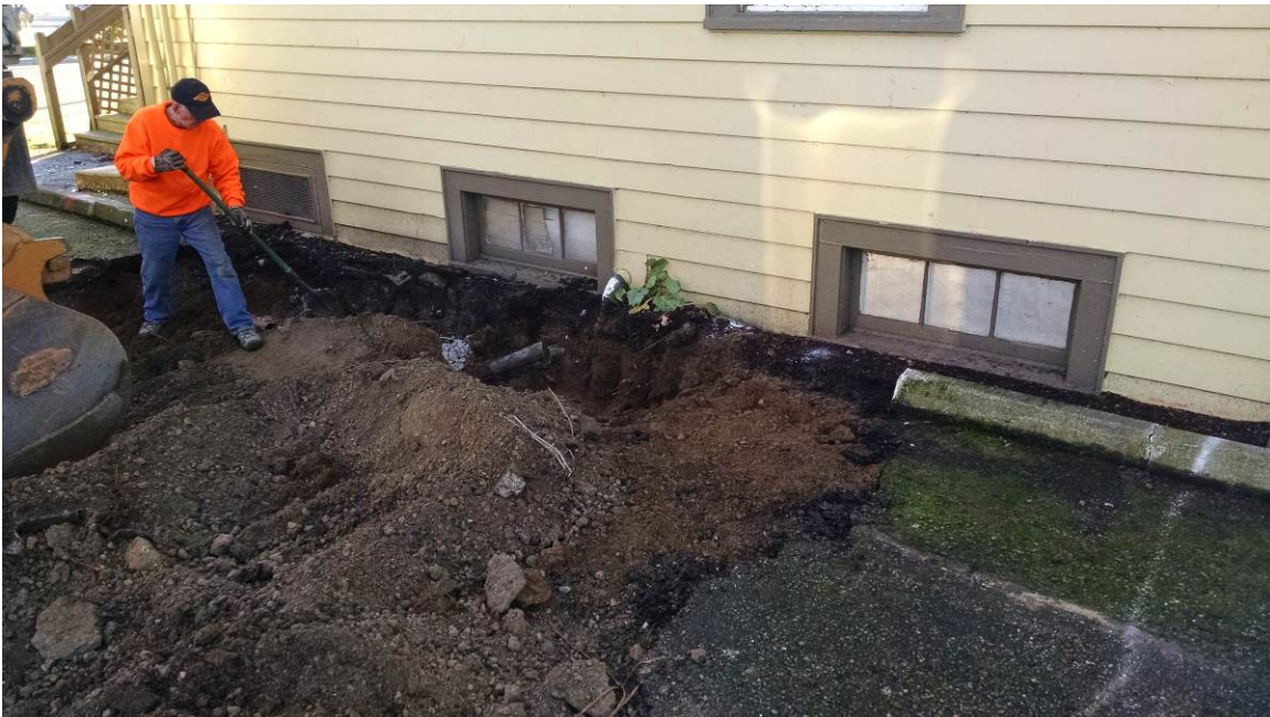
Photograph 3 – Removal of asphalt and grease trap. Grease trap/sewer piping visible by building foundation.
