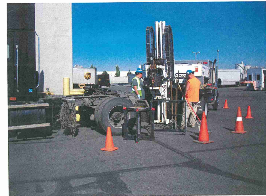
Photograph No. 2: View of sampling rig set-up on SB-01 locations. Former used oil/new oil UST pit was to the left, under the parked truck.
