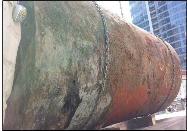
Removal of 1,750 gallon diesel UST. A hole is visible near the tank bottom – looking north
