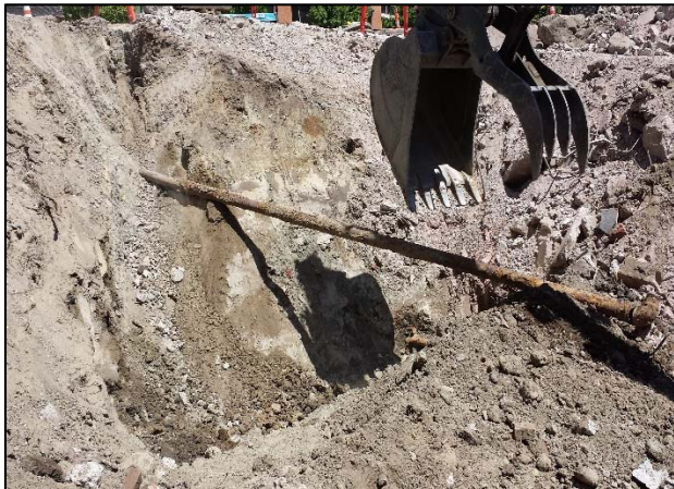
Excavation and removal of fuel supply line east of UST – looking southeast
