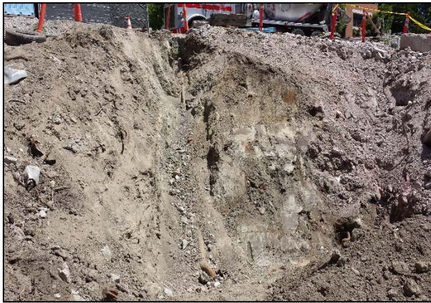
Preparing to remove the fill port (uphill), fuel supply line, and UST (downhill) in northeast portion of the Subject Property – looking east
