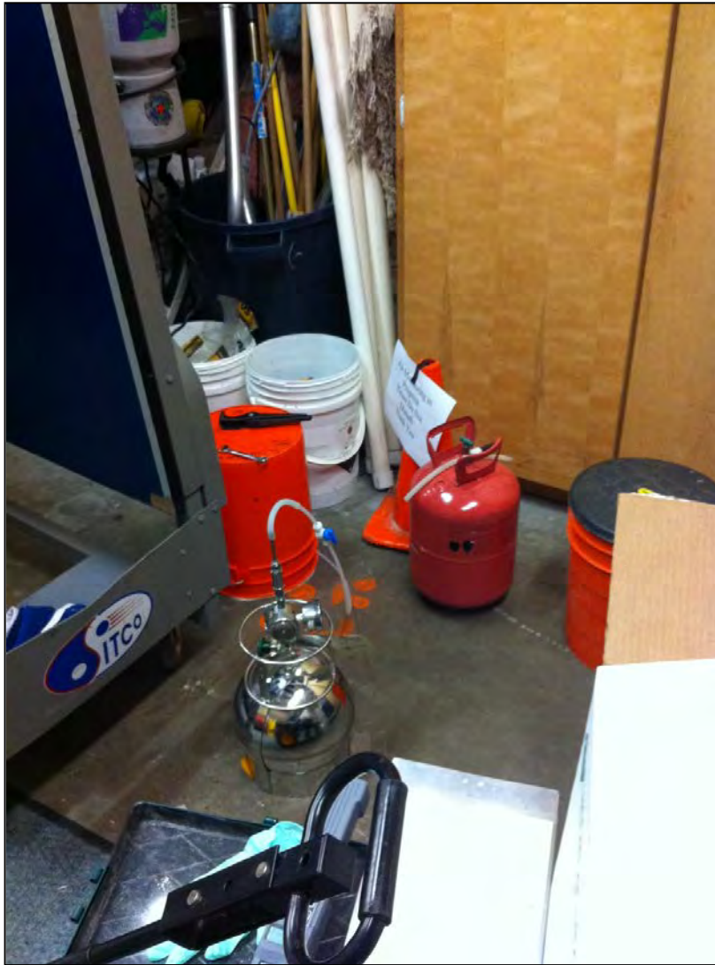
17. Sub-slab soil vapor (i.e. soil gas) sample SSV48 at YMCA collected in storage room.
