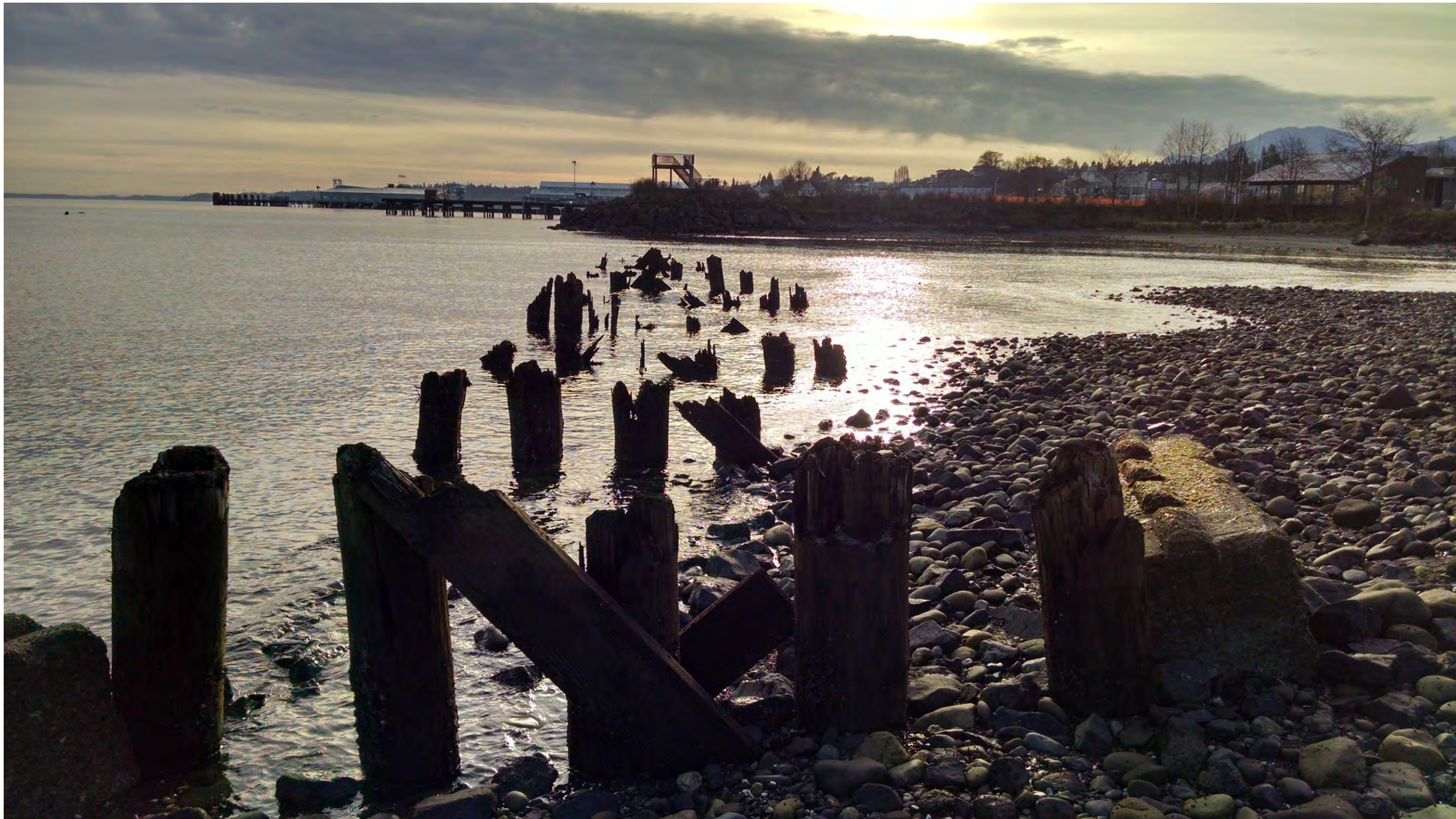
Photo D-4 – Trestle piles at Valley Creek estuary looking east. Bent, or pile group, spacing is about 15 feet on center. Each bent contained 5 to 6 piles spaced about 2 feet on center.
