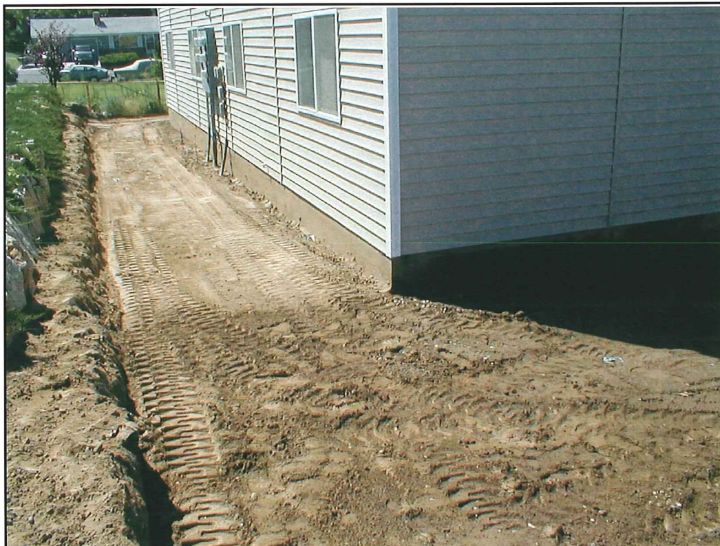
Photo 4: View of northeast corner of site after excavated to 12-18 inches below grade.
