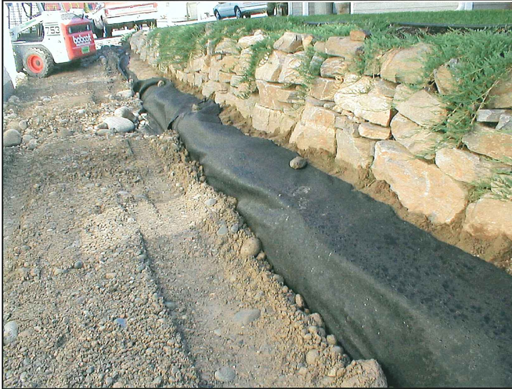
Photo 7: Edge of geotextile at eastern perimeter after 12 inches of gravel fill placed.
