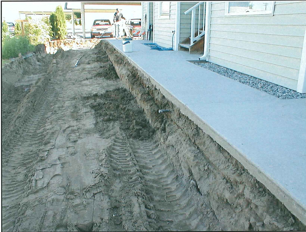
Photo 3: North-facing view of western perimeter after excavated to 18 inches below grade. Trench along western perimeter excavated to 36 inches below grade.
