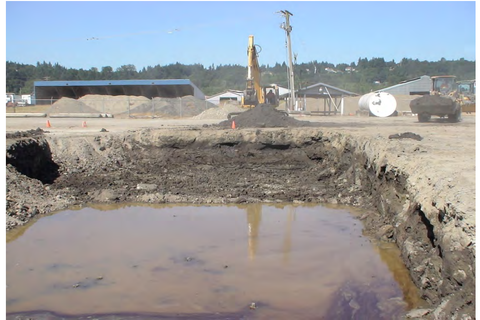
Dike at west end of excavation keeping floating DRO out of bench area.
