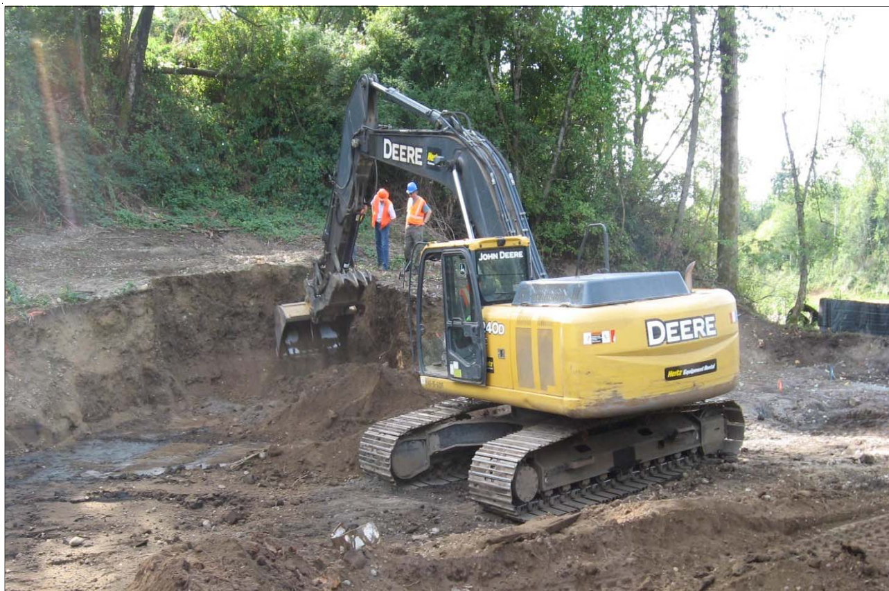
Removal of soil and landfill debris at Eldridge Municipal Landfill site (September 2011).
