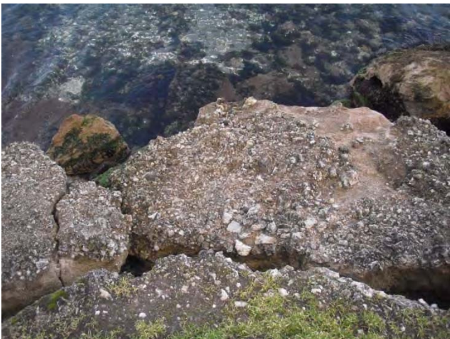
Photograph 5. Slag to Potentially be removed
