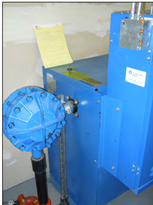
Photograph 18: Looking at the hydraulic oil reservoir for the elevator.
