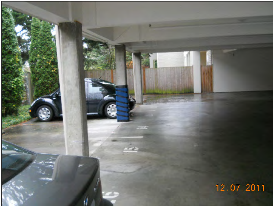
Photograph 19: Looking south into the street level parking on the northeast corner of the building.
