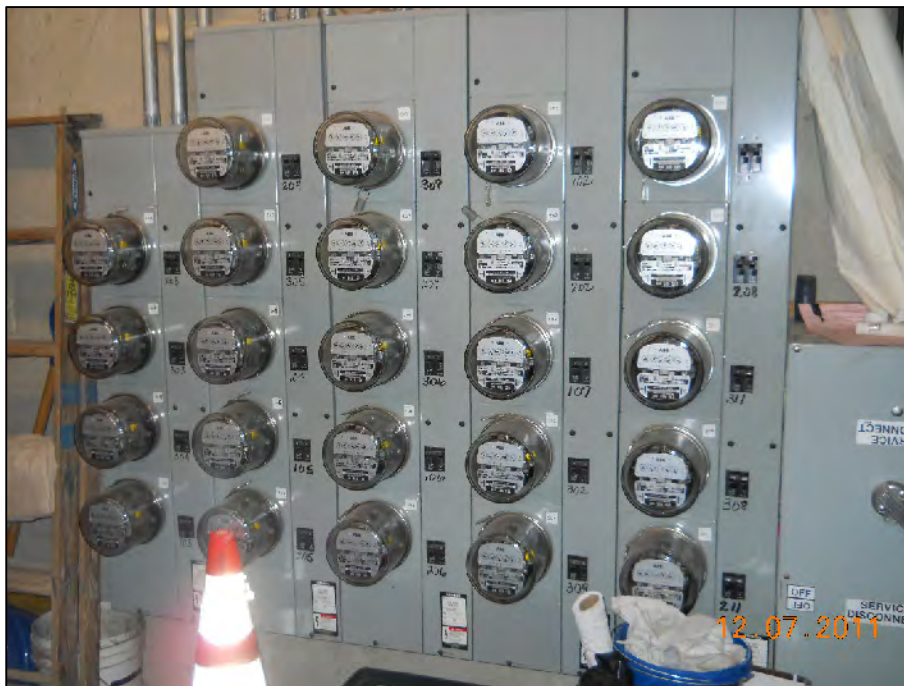
Photograph 16: Electrical meters on south wall of basement.
