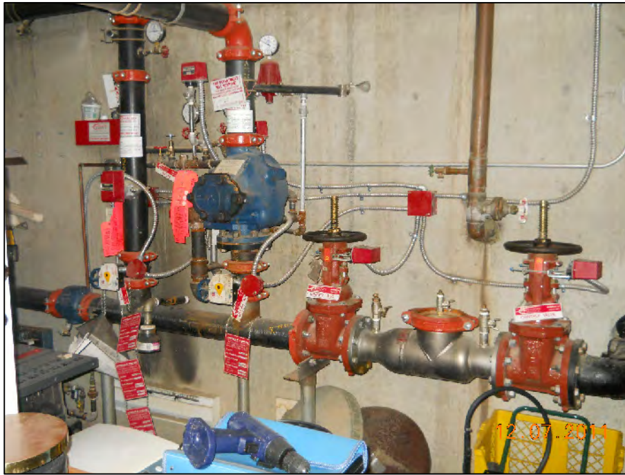
Photograph 15: Sprinkler system on west wall of basement, in maintenance shop.
