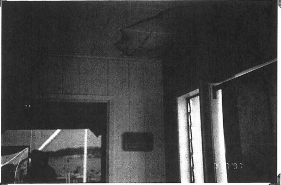
Viewing acoustical ceiling tiles (w/ dots) in front office portion (NW corner) of building. 7-17-97
