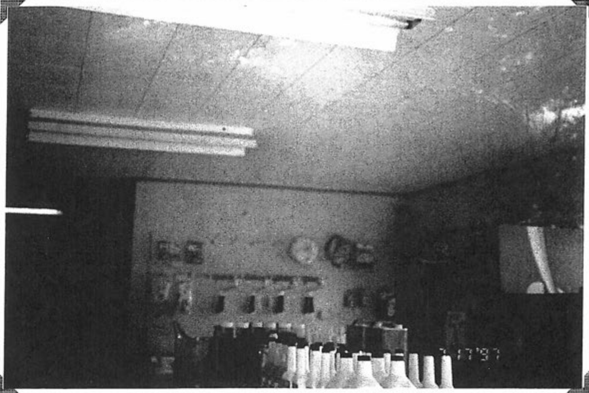
Viewing acoustical ceiling tiles (w/ smooth surface) in retail (front) portion of building. 7-17-97
