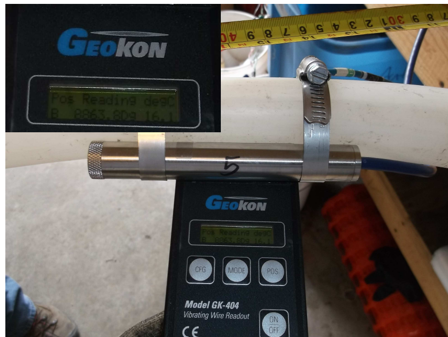
CASING BENT 16 INCHES FROM STRAIGHT
