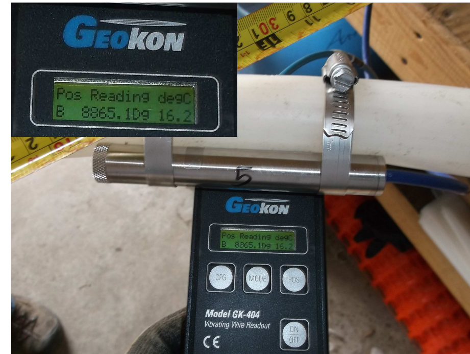
CASING BENT 12 INCHES FROM STRAIGHT
