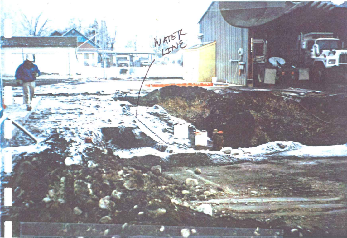
Photograph No: 1 UST excavation upon arrival. The diesel fuel UST had been removed prior to approval.
