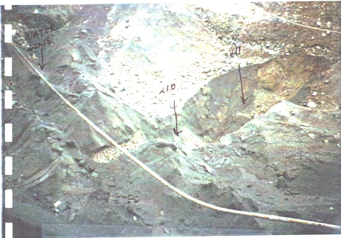
Photograph No. 2: Bottom of UST excavation. Sample locations for #PPC-3198-210 and 211. Bottom of diesel fuel UST and gasoline UST #2.
