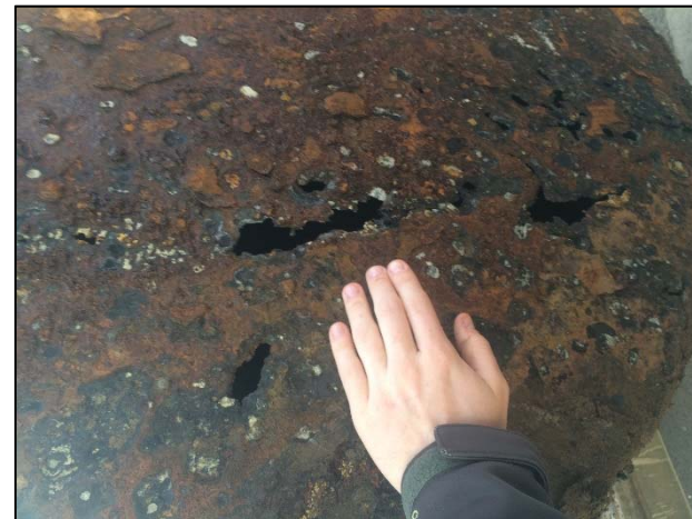
Photo 4. A close up view showing the poor condition of the bottom of the western tank's northern end.
