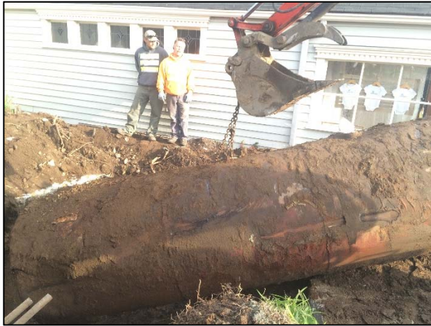
Photo 1. A view looking north at the removal of the eastern tank from the tank pit.
