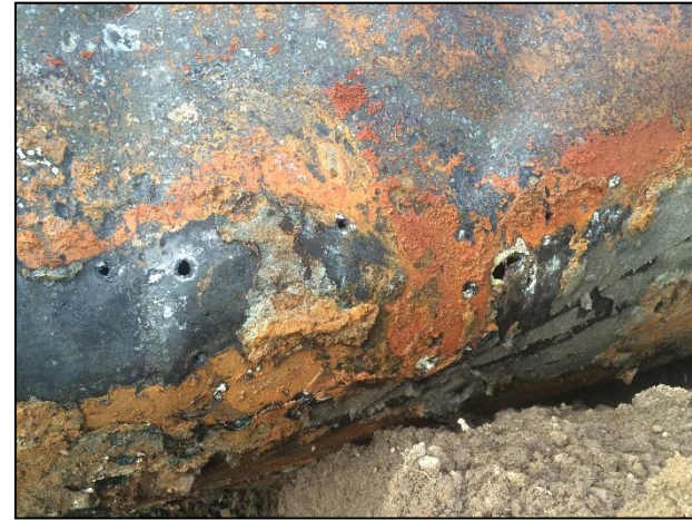
Photo 2. A view of the eastern tank showing the quarter sized holes as well as corrosion along the bottom of the tank.
