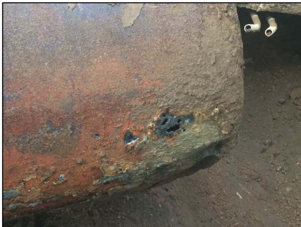
Photo 3. A view to the south of the bottom of the western tank along its southern end. Note the corrosion and several holes.
