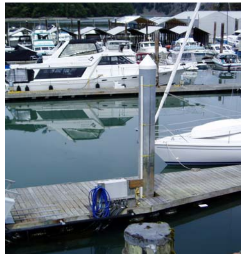
PVC Pipe on Dock Piling for Level Troll ® Protection
