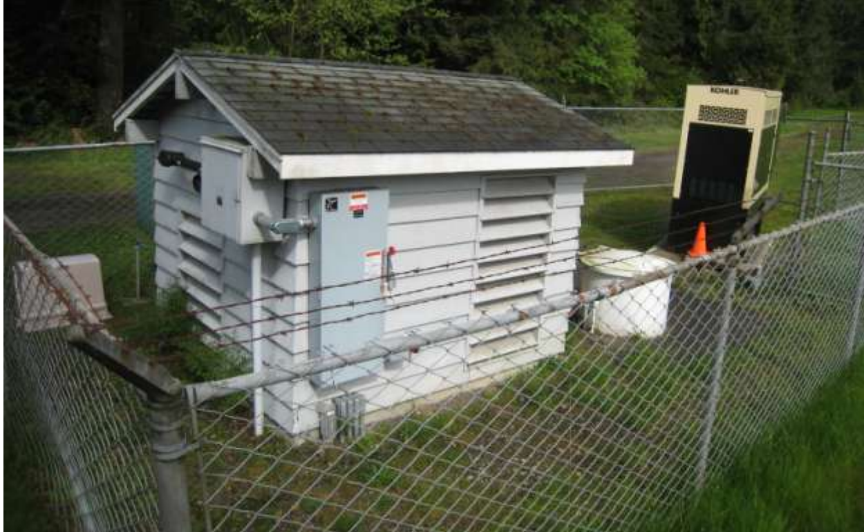
Photo 3: Lift station for sewer system adjacent to the Site, scheduled for replacement
