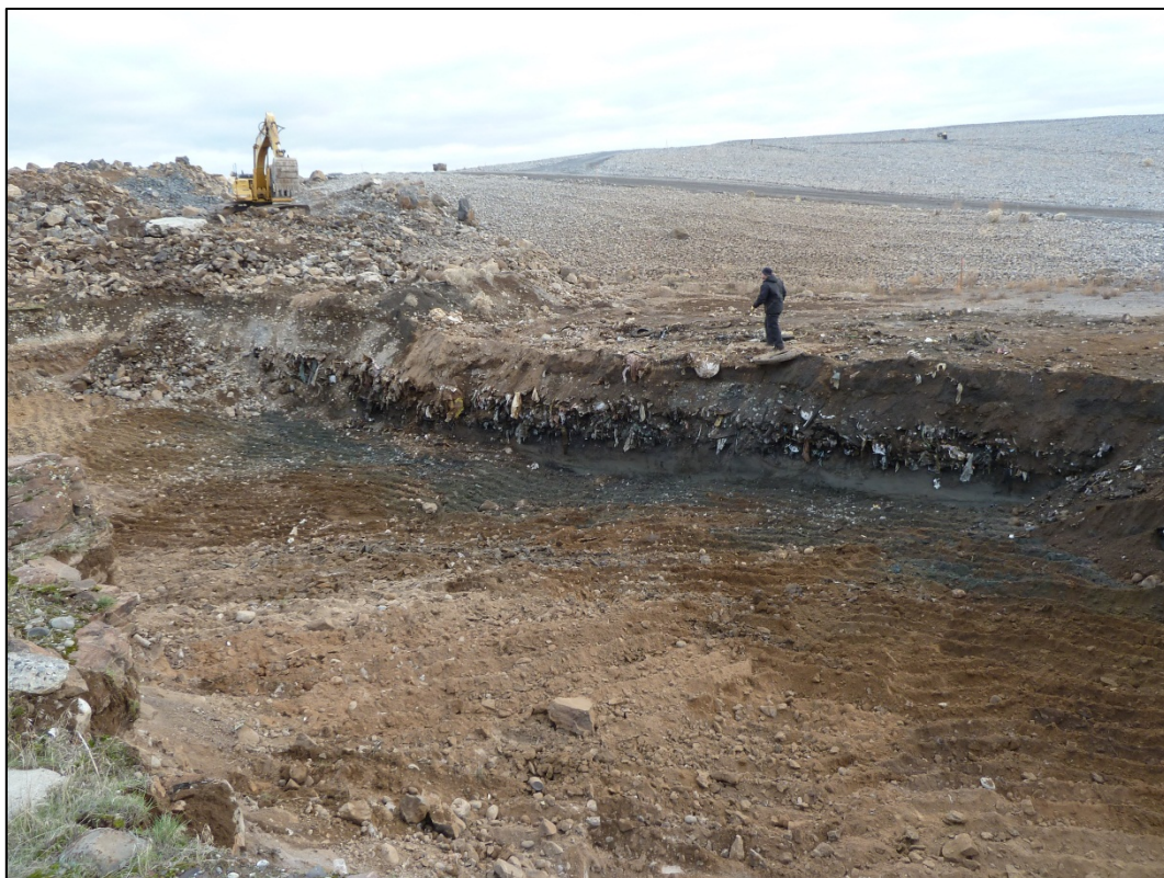
Photo 2: Refuse in eastern part of excavation (looking south):
