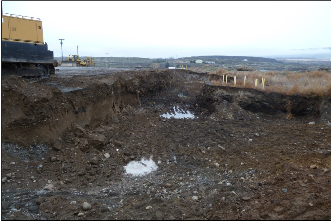
Photo 5: Area of saturation near MW-41a (looking west)
