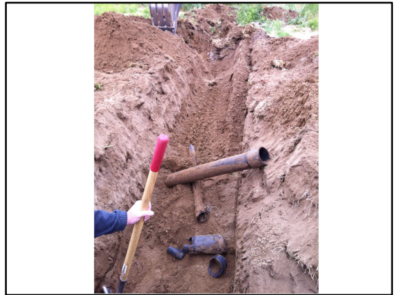
F. Old septic system pipe line (Orangeburg).
