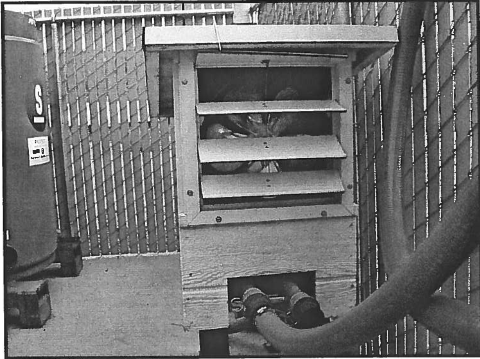
SVE blower within ventilated housing.
