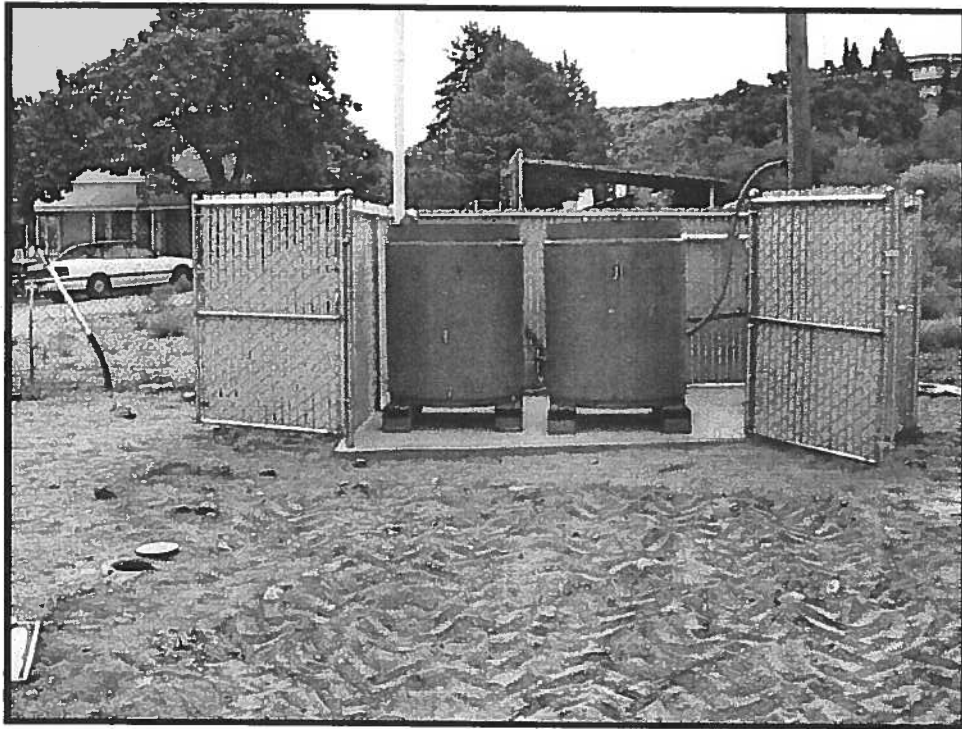
Carbon-filled canisters inside system enclosure (west to east view).
