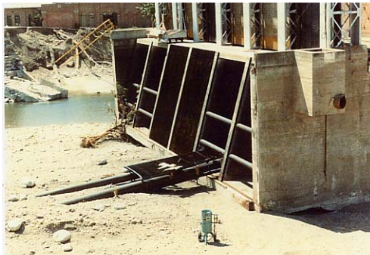
Photo 3. Channel Erosion adjacent to Powerhouse Intake
