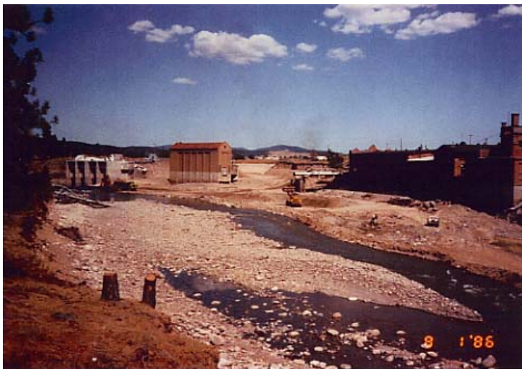
Photo 2. Powerhouse and Bank Erosion from Downstream
