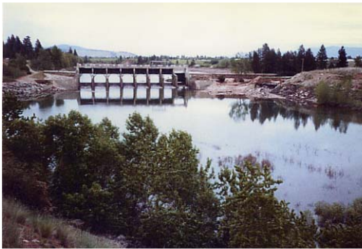
Photo 5. Erosion at Upriver Dam from Downstream
