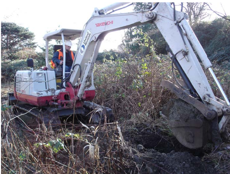
Small track excavator used to excavate test pits. Reconnaissance test pit RTP-13 is shown in the photo.
