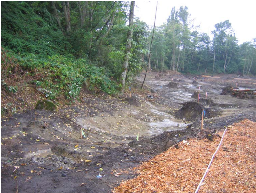
Confirmation sampling locations at base of new BTC/Birchwood channel and eastern sidewall/slope.
