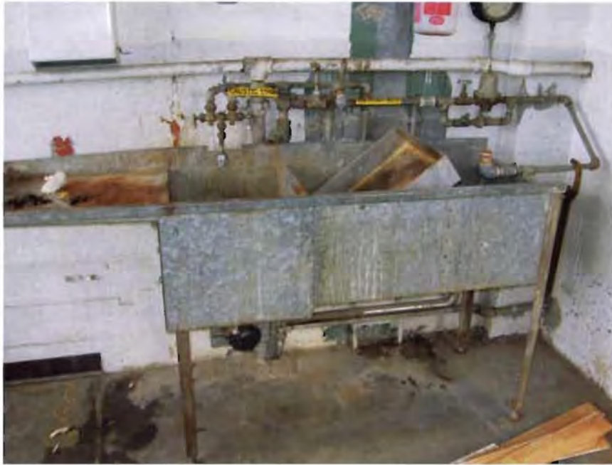
Photo 27 – Cleaning area in maintenance shop in southern portion of building main floor.
