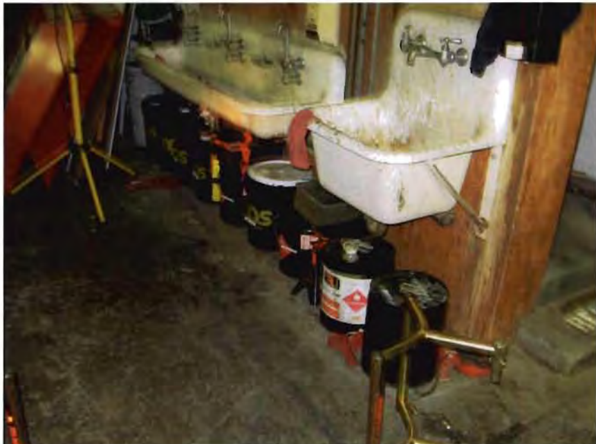
Photo 20 – Oil and fuel container storage in northern portion of basement.
