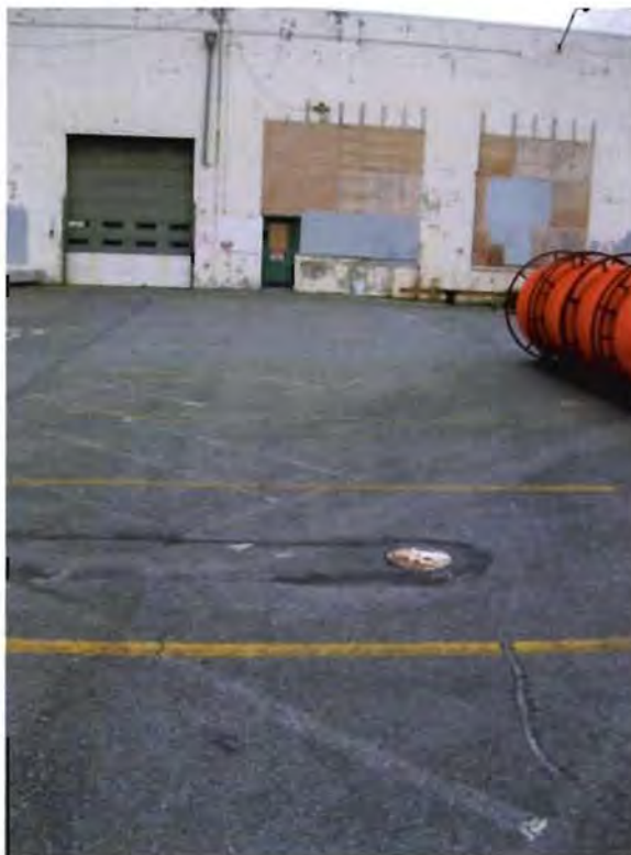
Photo 3 – Possible vapor extraction well head in parking lot at north end of property.
