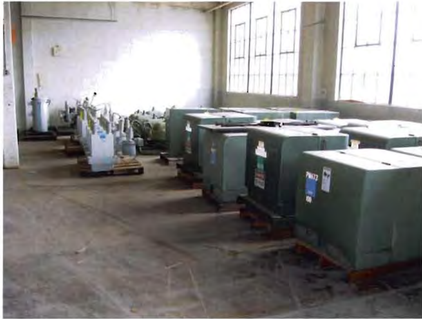
Photo 25 – Transformer storage in central portion of building main floor.
