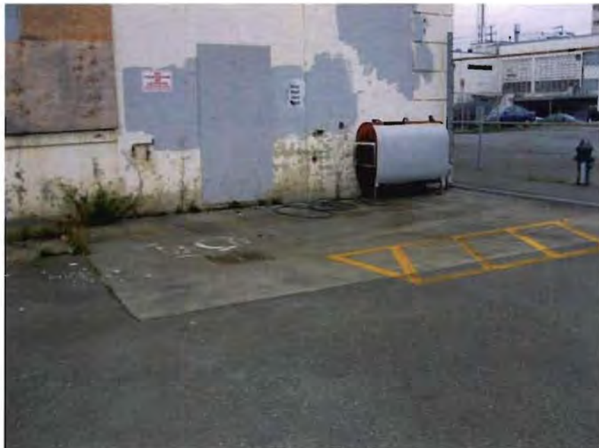
Photo 10 – Aboveground oil storage tank and wash down area at north end of property.
