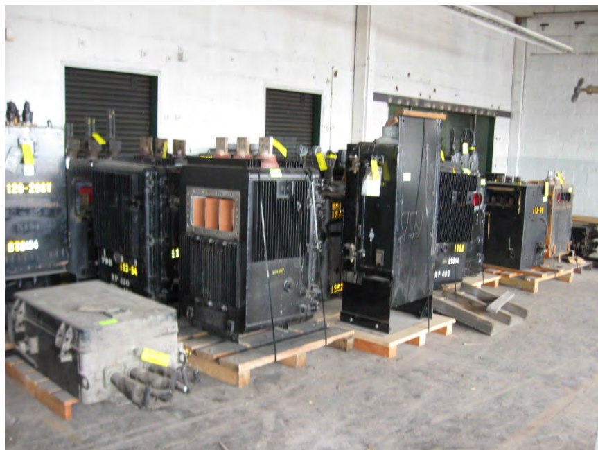
Photo 24 – Transformer storage in central portion of building main floor.
