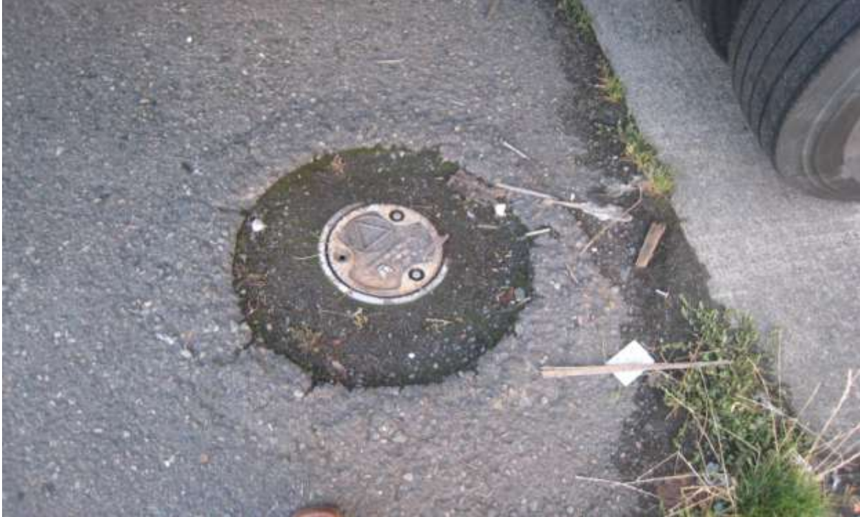
Photo 3: Monitoring wells are still in use at the property
