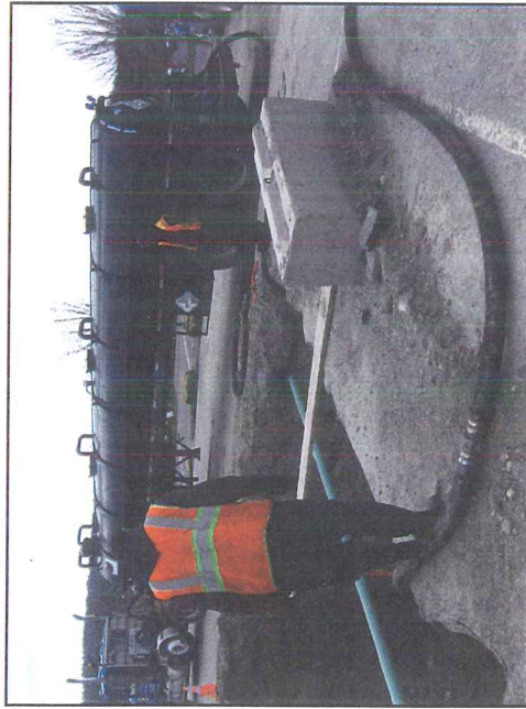
Photograph 3. A view to the south of MarVac Services removing pit water from the western tank pit prior to excavation of PCS.
