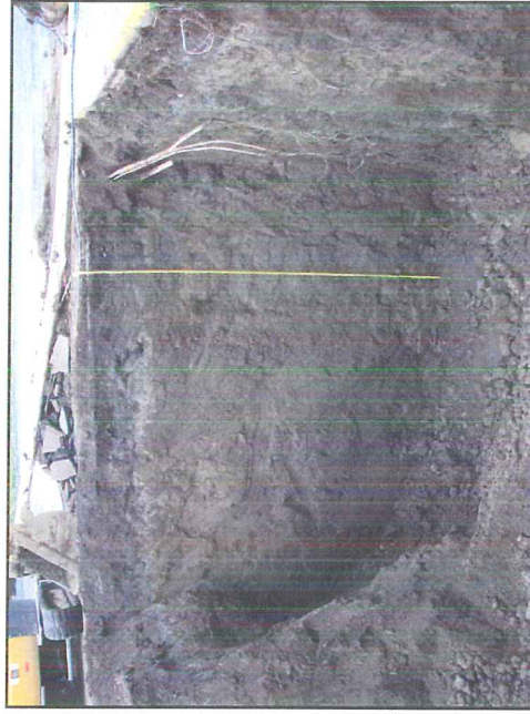
Photograph 4. A view to the west looking at the western tank pit west sidewall. Note the dry silt and no evidence of groundwater recharge.
