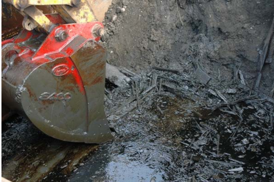
Photo 9. Wood debris in excavation
