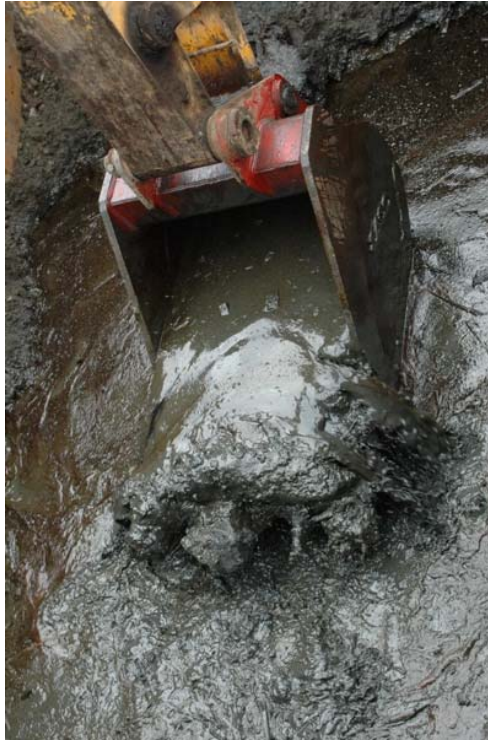
Photo 11. Slurry created by agitation of native silt unit
