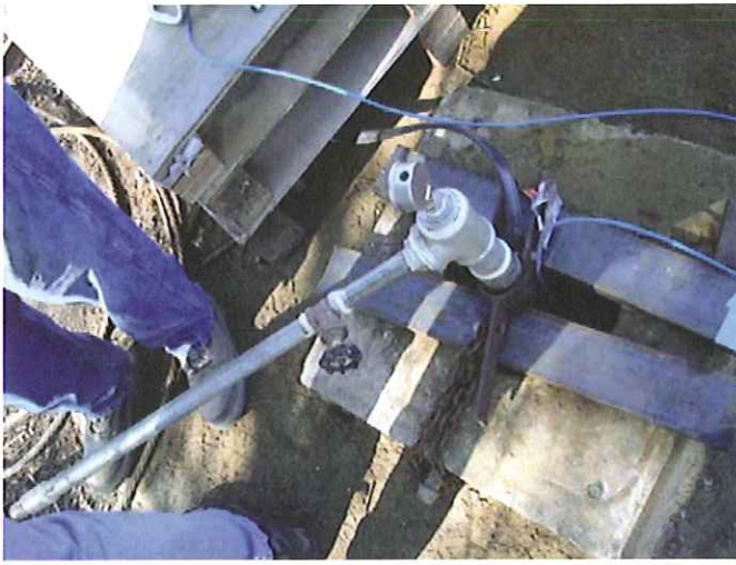
Photograph 7. Active production well during pump testing on the southeastern portion of the WHC Property.
