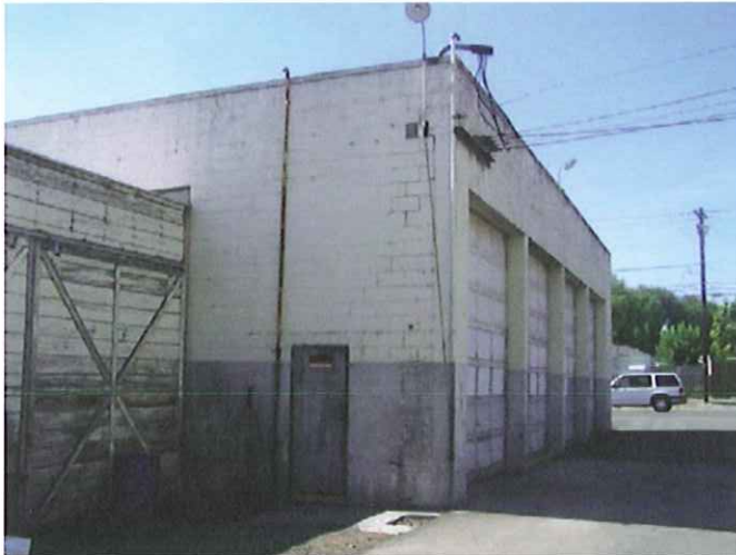
Photograph 15. Vent lines on the exterior of the truck maintenance facility on the WHC Property. Photo facing west.
