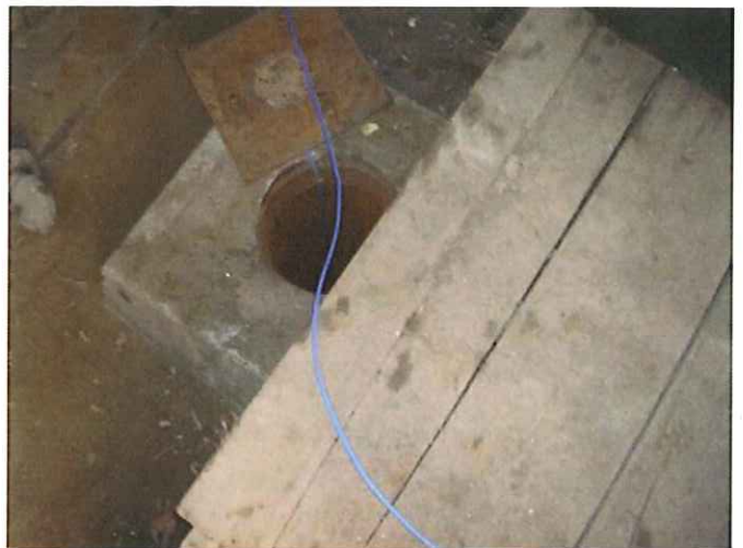
Photograph 6. Production well located in the WHC building.
