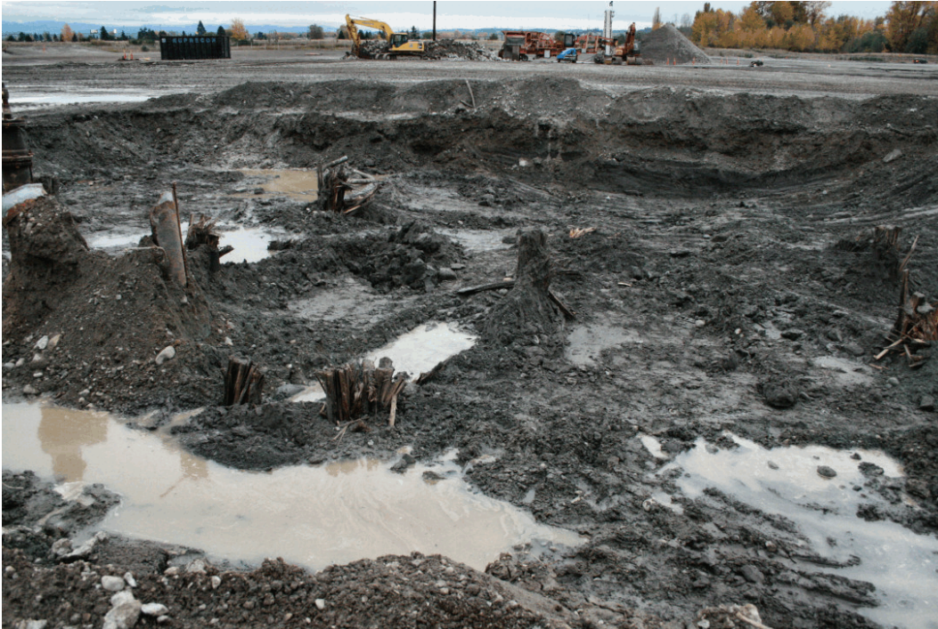
30. View of the middle section of the hydraulic area excavation on November 11th.
