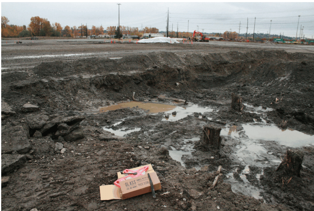
29. View of the eastern end of the hydraulic area excavation after rain on November 11 th . The tops of the wood pilings from the sawmill building are exposed.
