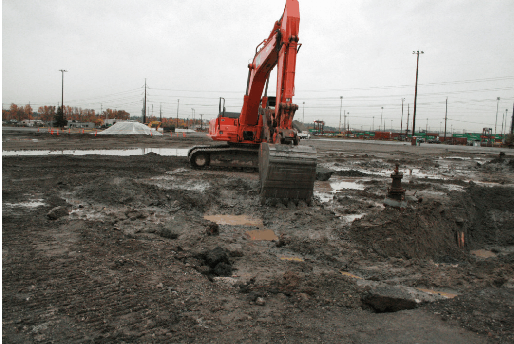
28. View of the trackhoe beginning excavation in the hydraulic equipment area of the sawmill.
