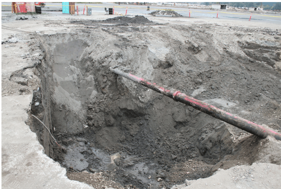
11. View of the excavation west of the fire line, which remained unsupported during the digging.
