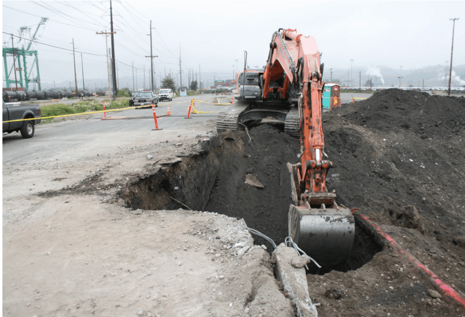
10. View of the trackhoe excavating oily soil from the area to the west of the fire line.
