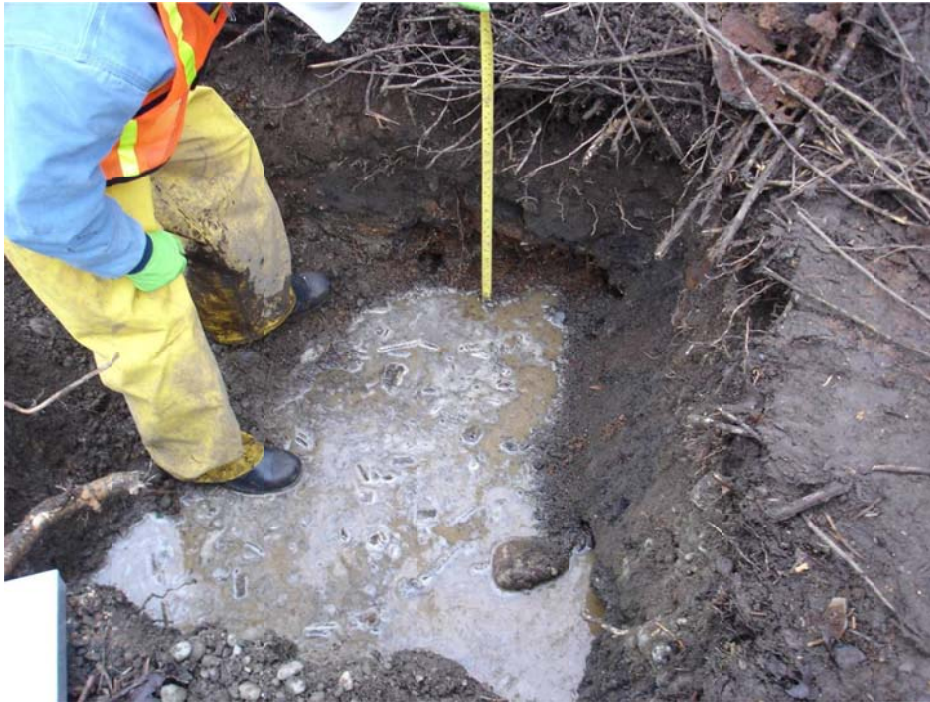
TP-22 West Sidewall
