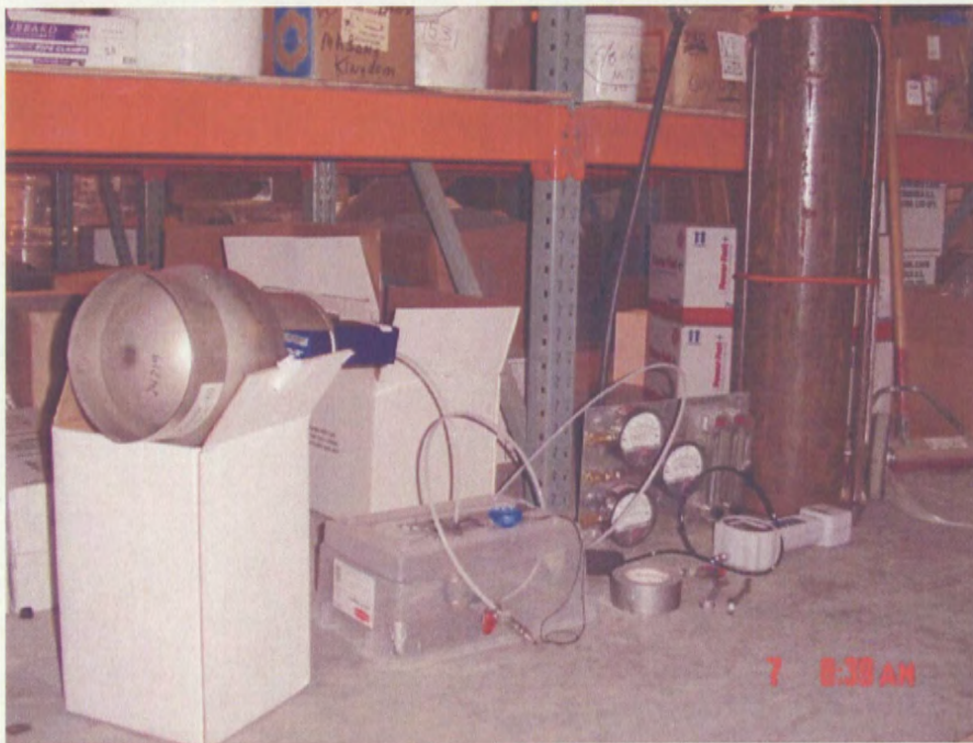
Sub-slab Sample Location V-3 – Sampling Setup
