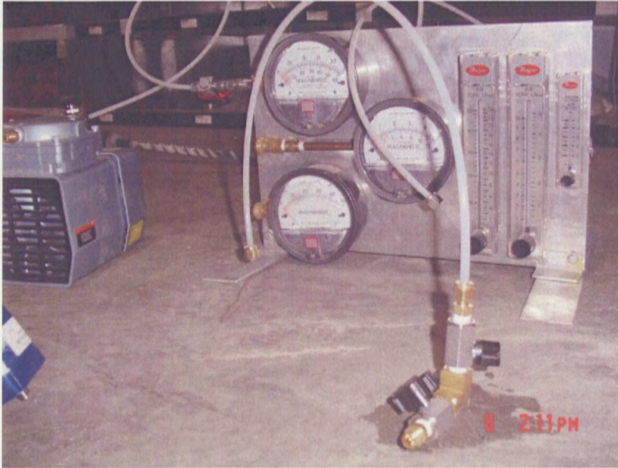
Sub-slab Sample Probe and Gauges
