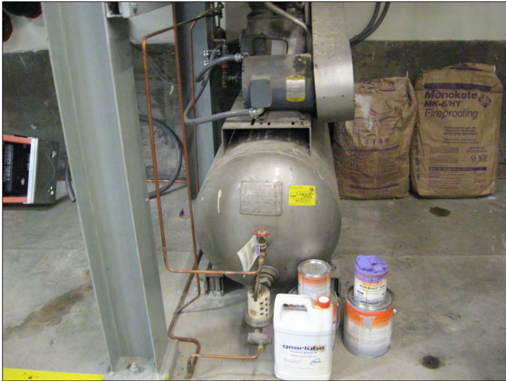
2. Air compressor on lower level of Building 18-03.
