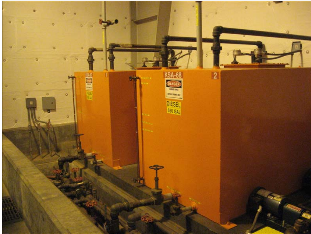
3. ASTs KSA-67 and KSA-68 in Building 18-11.
