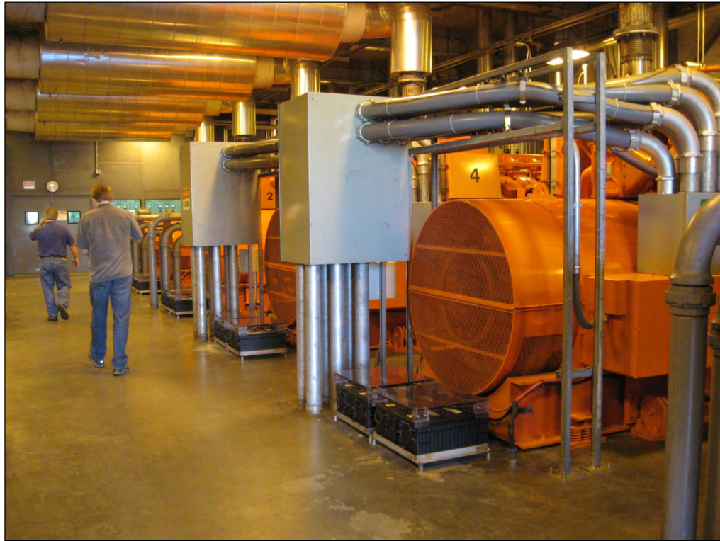
5. Diesel generators and associated batteries in Building 18-11.
