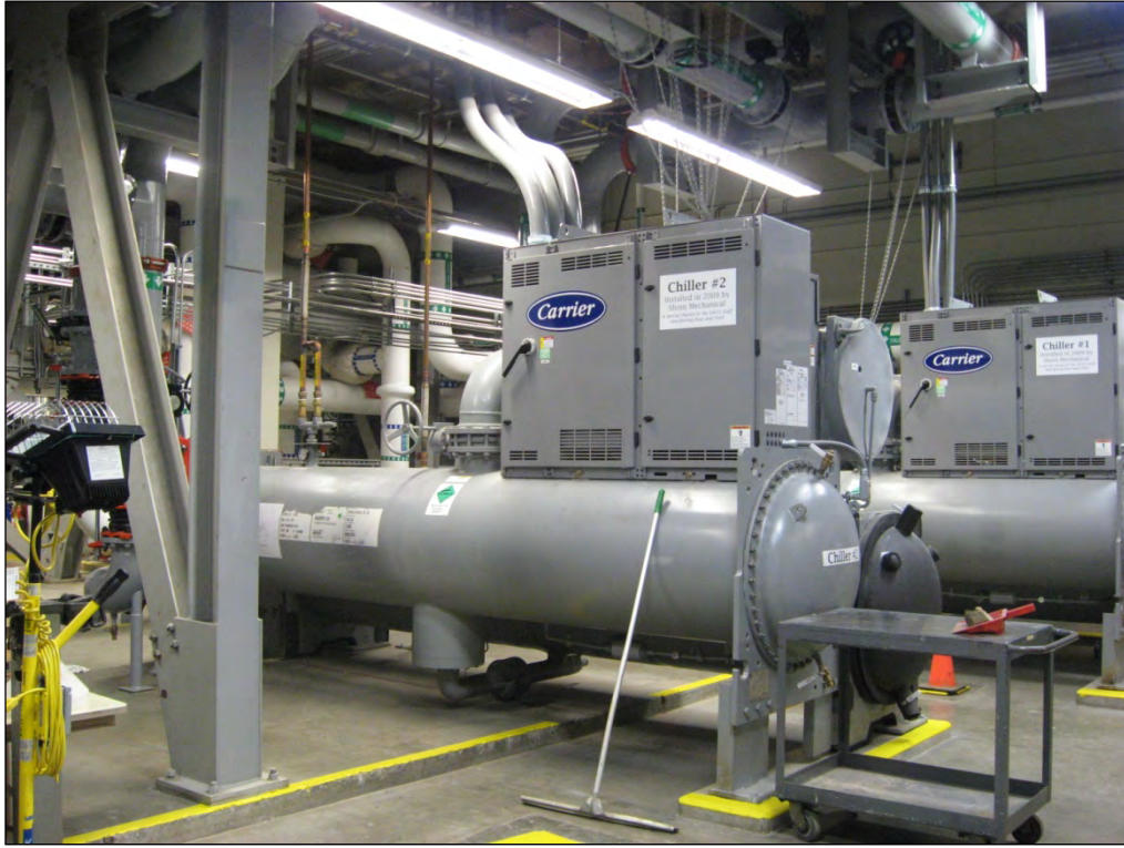
1. Chillers on lower level of Building 18-03.
