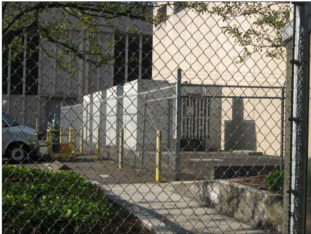
8. Oil-filled electrical transformers east of Building 18-11.
