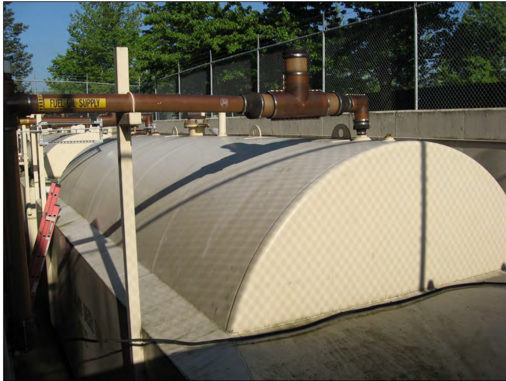
7. ASTs KSA-71 and KSA-72 north of Building 18-11.
