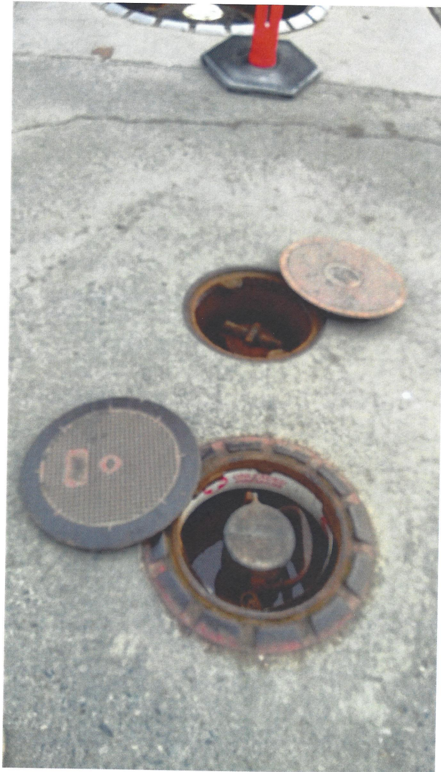
Picture 3. Fill port where spill occurred filled with gasoline.
