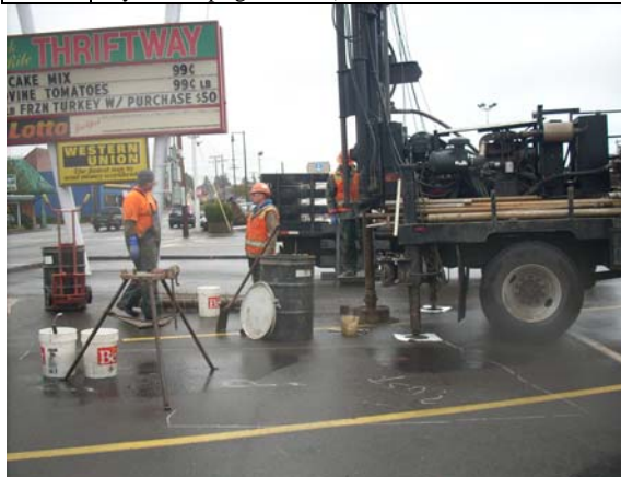
Photo #5: View of hollow stem auger drilling at MW-1, adjacent to potential abandoned fuel tank (outlined in foreground) at former Flying A gas station. View looking to the east.
