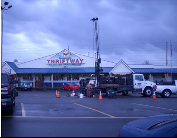
Photo #7: View of drilling at boring MW-4, adjacent and southeast of potential abandoned fuel tank at the Site. Photo taken facing south.
