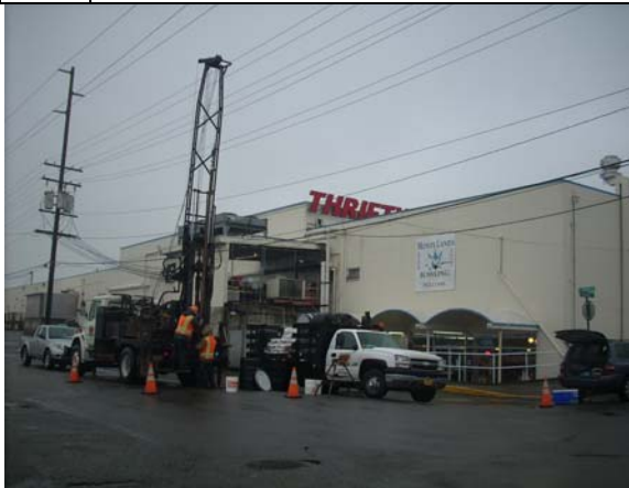
Photo #11: View of drilling at boring MW-10, in the City's right-of-way on Wynoochee Ave.. Boring is south of the Pick-Rite property. Note abundance of overhead power lines
