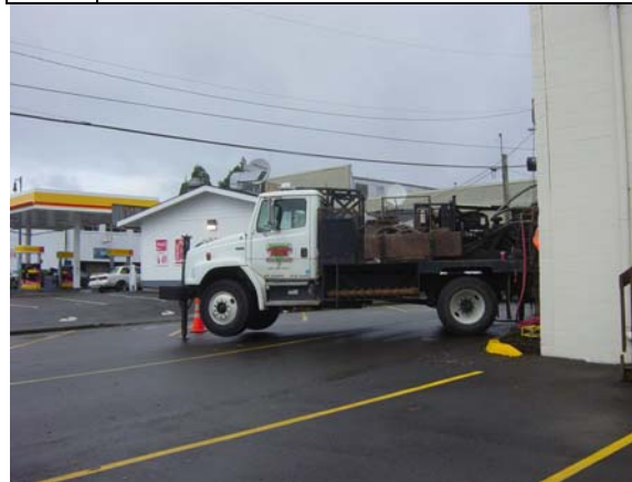
Photo #6: View of drilling at MW-2, southwest corner of Thriftway-Value Drug Building, along the alley of the City of Montesano sewer line/sewer lift stations.
