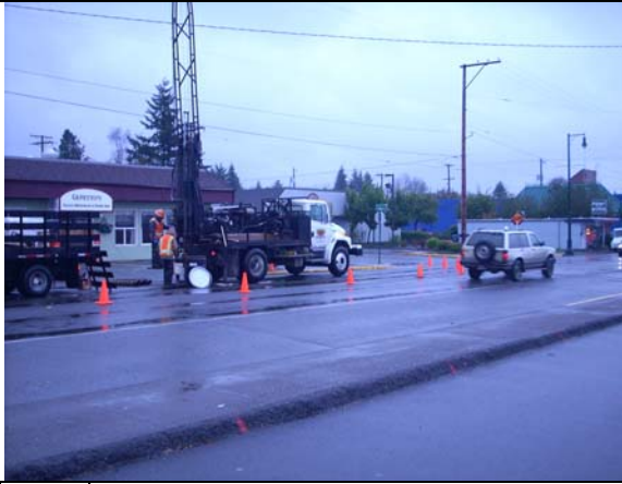
Photo #9: View of drilling at boring MW-6, adjacent south of a former gas station which is now occupied by Geppetto's Restaurant. Photo taken facing east.
