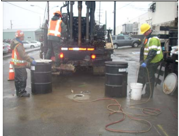
Photo #12: View of pumping and purging as the second half of mechanical development activities at monitoring well MW-10. Mechanical swabbing and surging was already completed.
