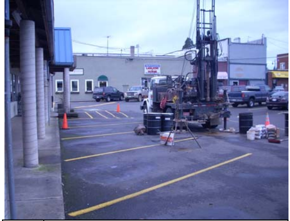
Photo #8: View of drilling at boring MW-5, adjacent north of the Pick-Rite Thriftway building, looking to the west.
