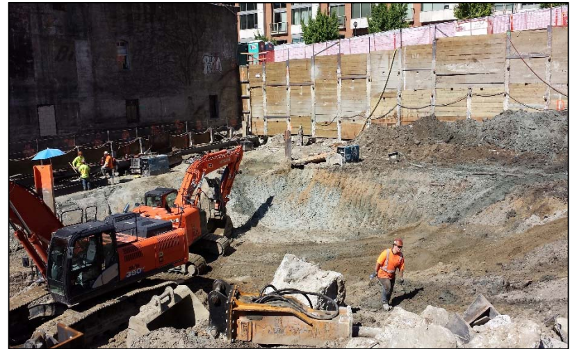
12. Clean native soil at the former elevator shaft and hydraulic hoist location in central portion of the subject property – Looking Northeast
