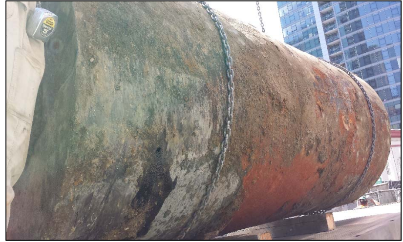
14. A small hole is visible in UST3 that was removed from the subject property
