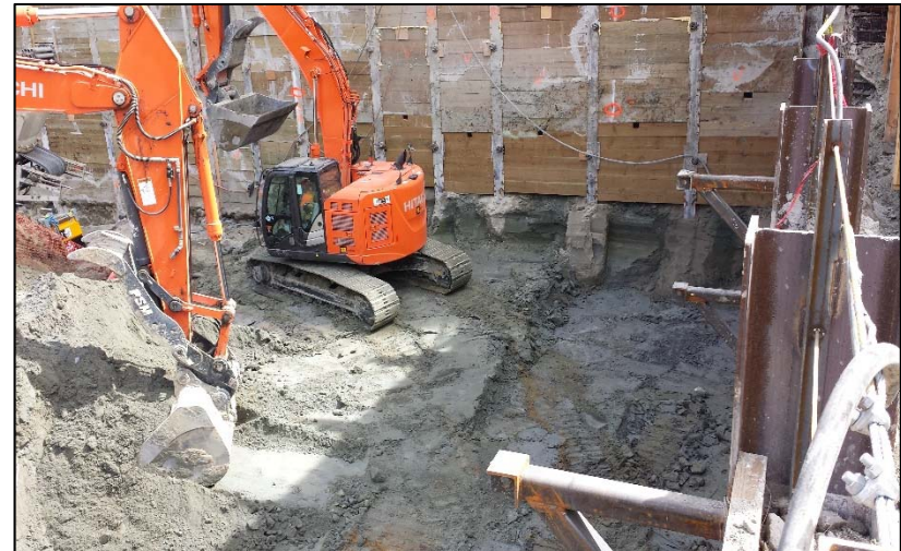
8. Clean native soil following excavation of contaminated soil at the former UST2 location in southwest portion of the subject property - Looking South
