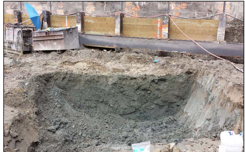
16. Clean native soil following excavation of contaminated soil at the former UST3 location – Looking North
