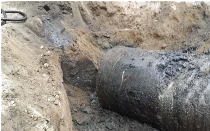
7. Controlled Density Fill inside the former UST2 and associated contaminated soil prior to excavation - Looking West
