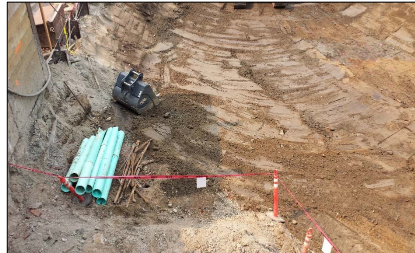
4. Non-contaminated soil underlying the contaminated fill soil excavated from the subject property - Looking North
