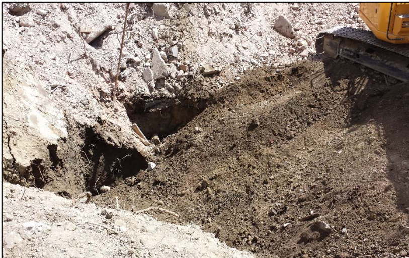
15. Contaminated soil at former UST2 location on the subject property
