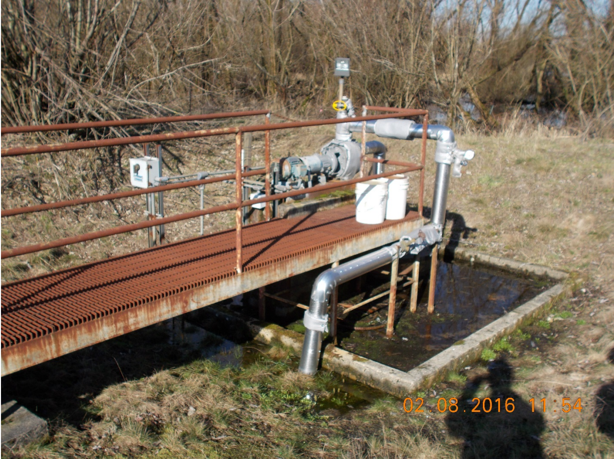
Photo 2: NIA Interception Trench Pump
