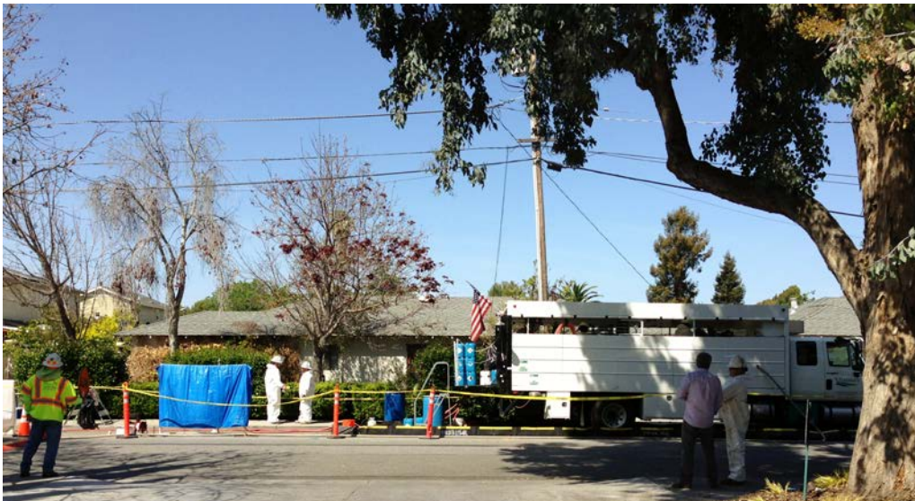
Image of similar groundwater injection set up. The white truck houses the injection equipment.
