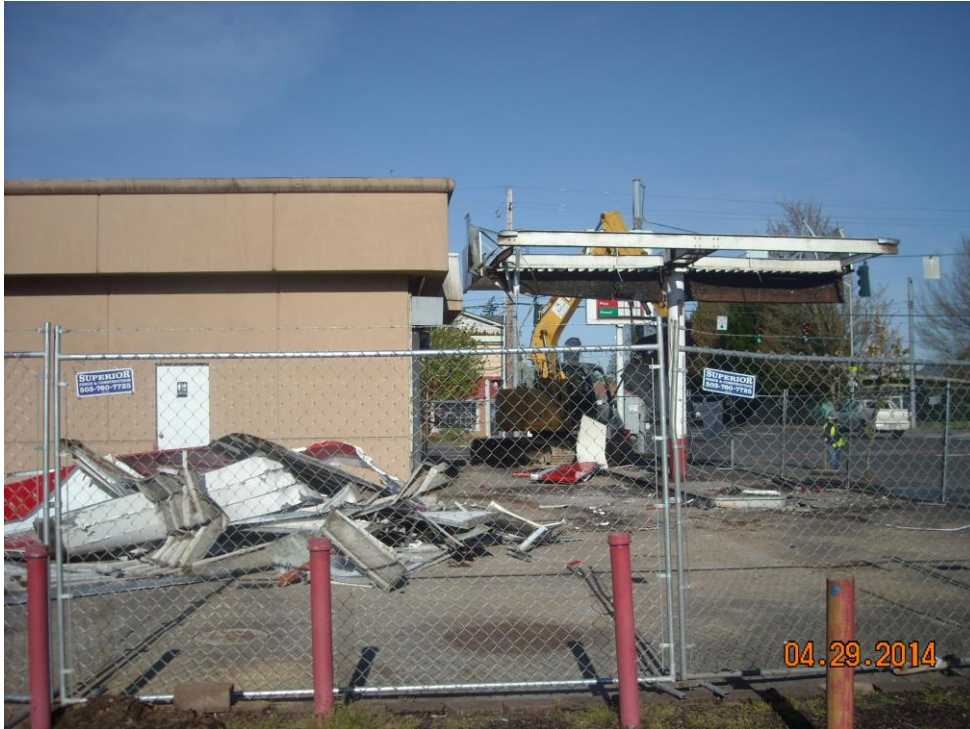
Photo 9 Looking west at convenience store building and dispenser island canopy (partially demolished). UST complex in foreground (center of complex below debris pile).
