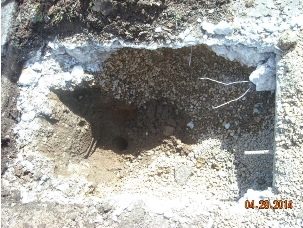
Photo 5 Looking into THE-6.5 sample location with typical surficial fill material in upper soil layer.
