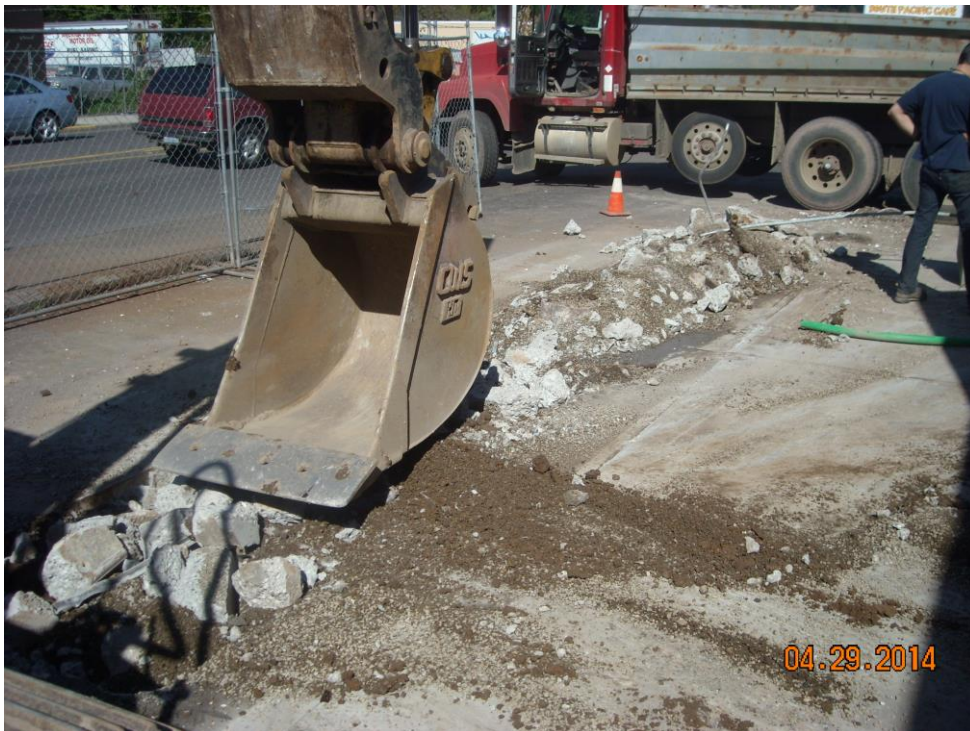
Photo 14 Looking northeast at dispenser island area, removing concrete debris in advance of collecting soil samples.
