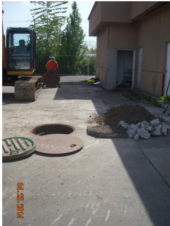
Photo 2 Looking south at THW-5 sample location on the west side of the UST complex.
