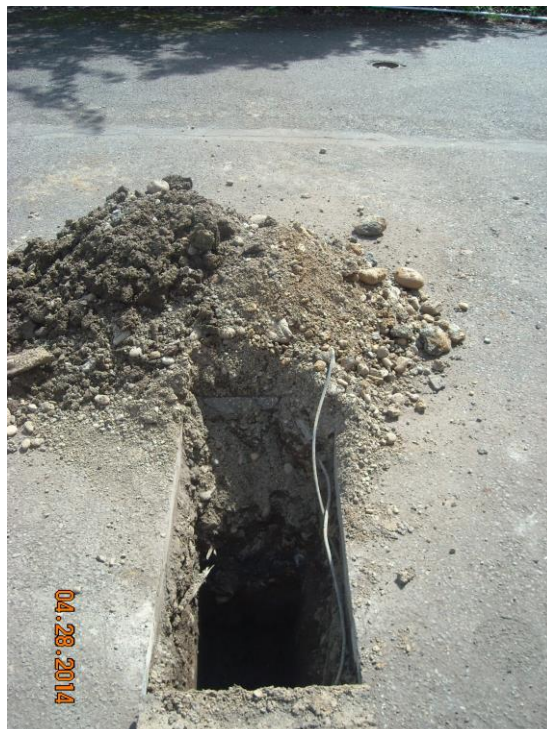
Photo 4 Looking south at THS-6 sample location on the south end of the UST complex.
