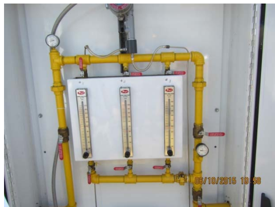
Natural Gas Flow Controls
