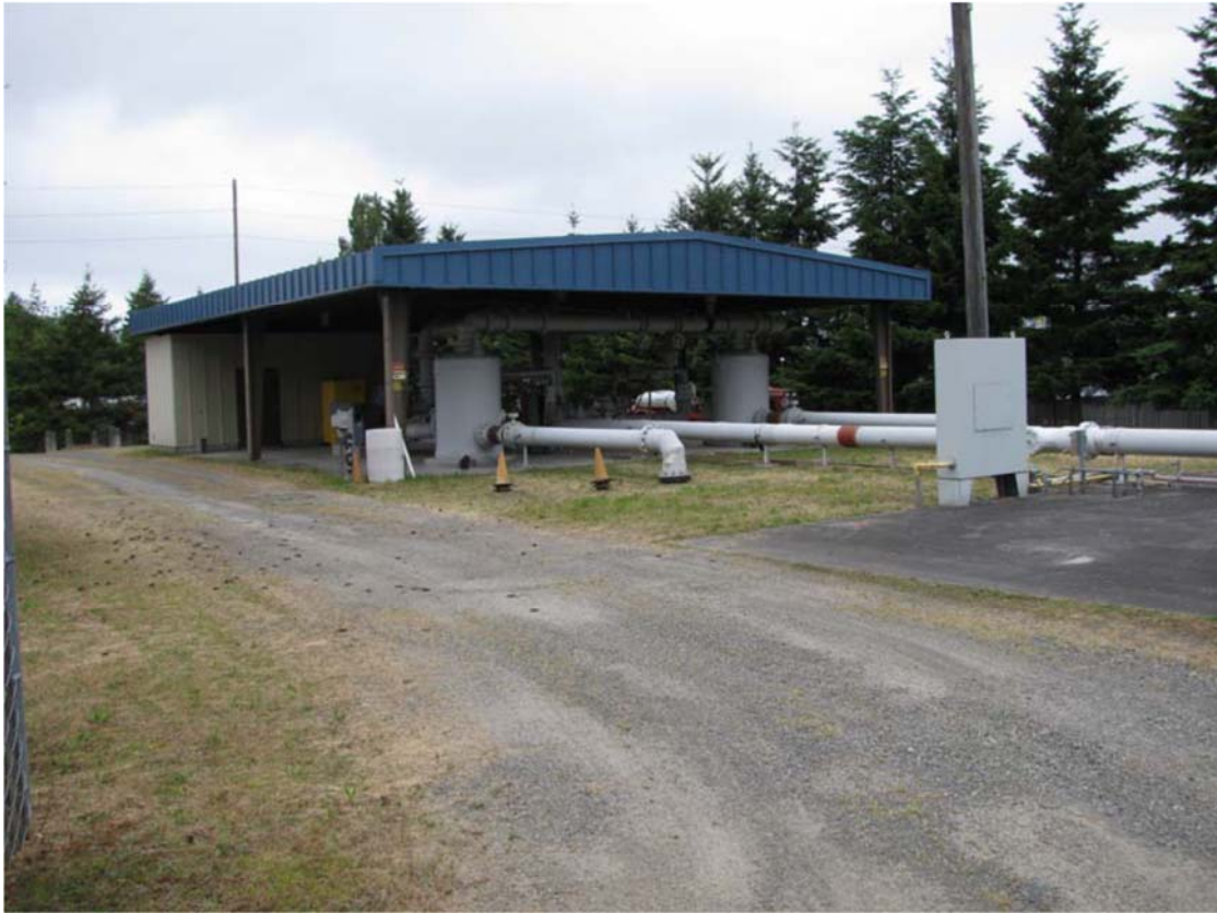
Landfill Gas Extraction System Mechanical Room
