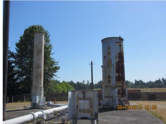
Landfill Gas Flares (current flare on left, backup on right)
