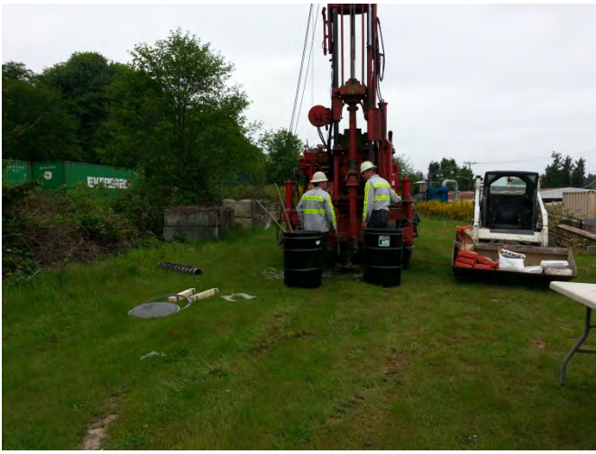
Photograph 7. Drilling on the BNSF Parcel in the vicinity of Former Rail Spurs #1 through #4 viewing southwest.
