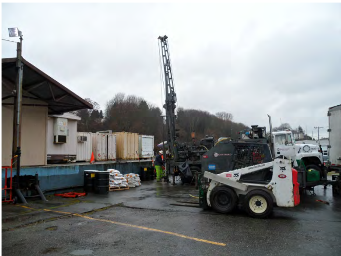
Photograph 5. Drilling in the vicinity of Former Rail Spur #1 and Former Barreling Shed #3 viewing southwest.
