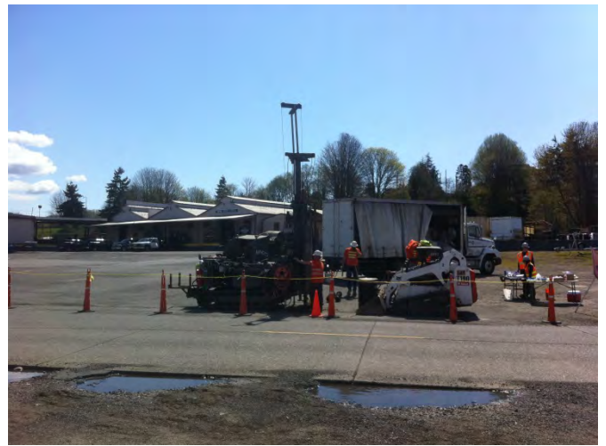
Photograph 6. Drilling on the south portion of the ASKO Hydraulic Property viewing north.
