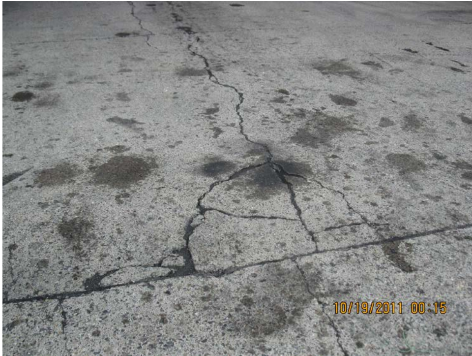
Photo 3: Development of Cracks on the Cap
