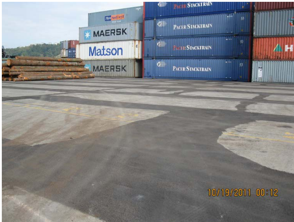
Photo 2: Typical Crack Repair and Containers Storage Area – from the east
