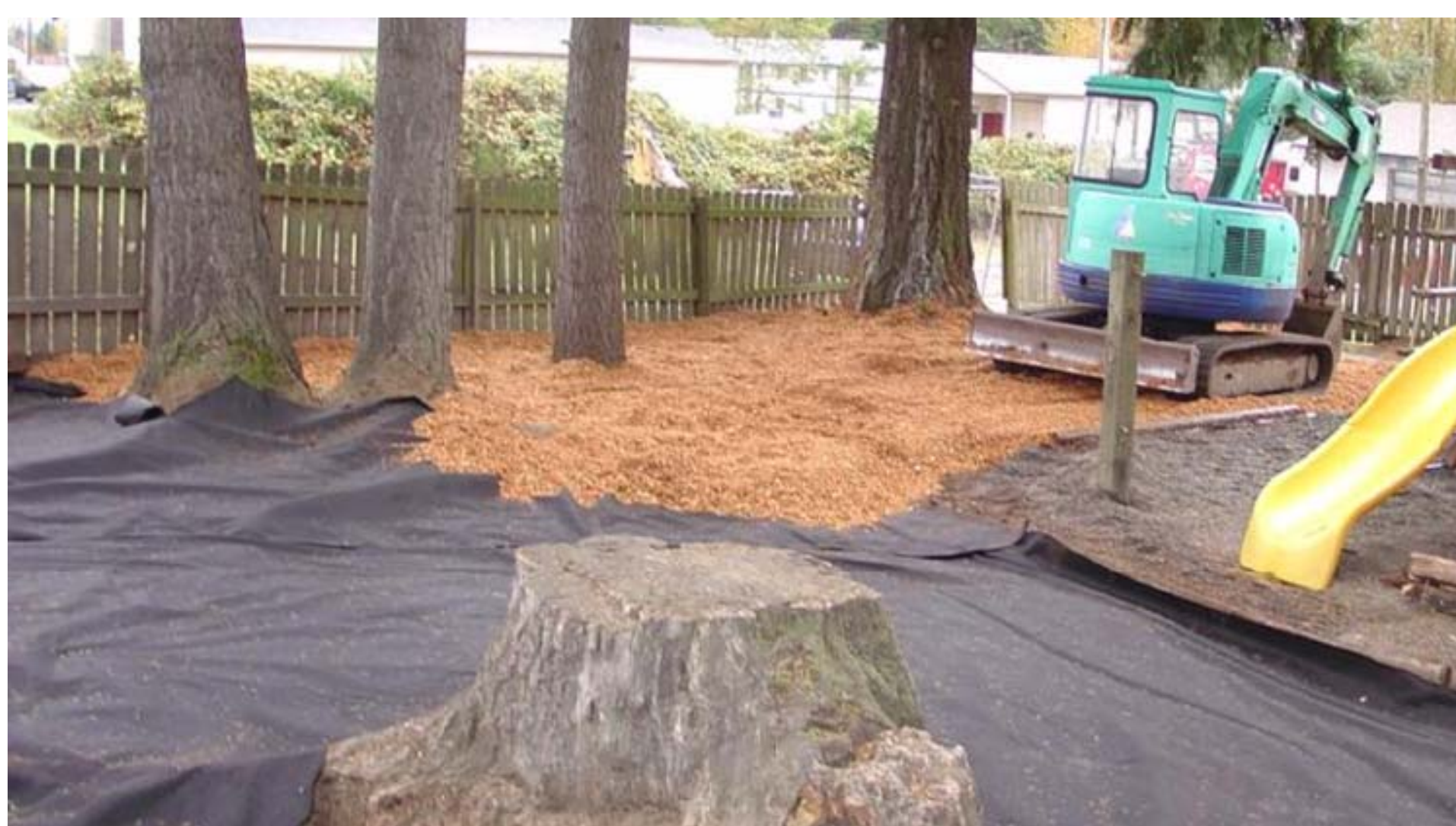
A fabric (like a thick weed barrier) covers contaminated soil. For yard cleanups, we will use a 24-inch soil cap.
