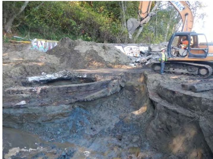
TPH Area excavation. From left to right showing second and first rows of kilns (Photo courtesy of SWCA Environmental Consultants)
