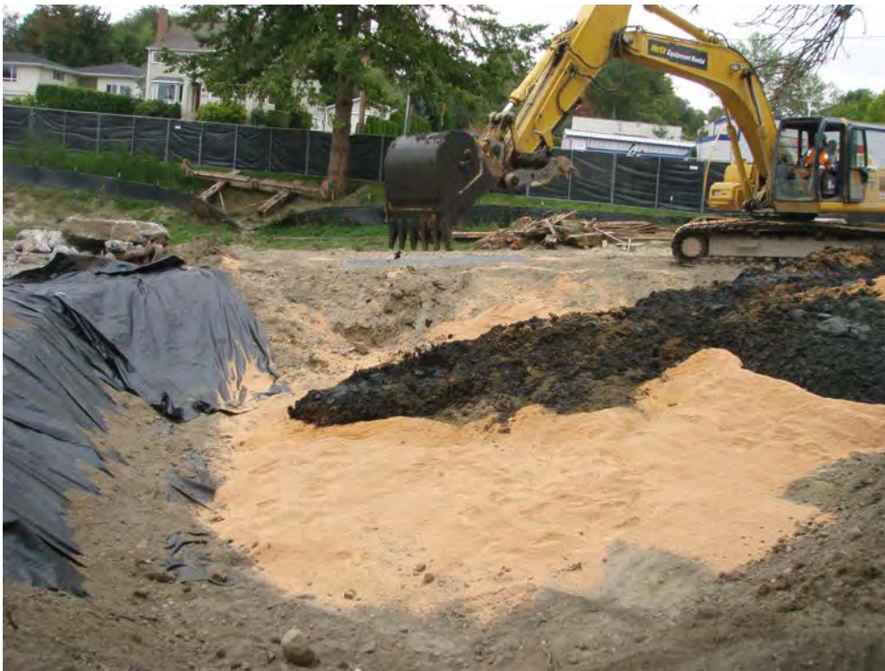
September 19, 2008. Upland mixing area where saw dust and sediment were combined to reduce free water for transport and disposal.
