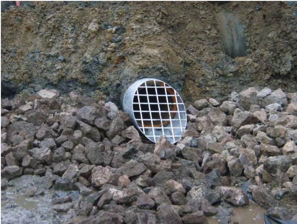
October 30, 2008. Construction and stabilization of the stream outlet at the new shoreline.
