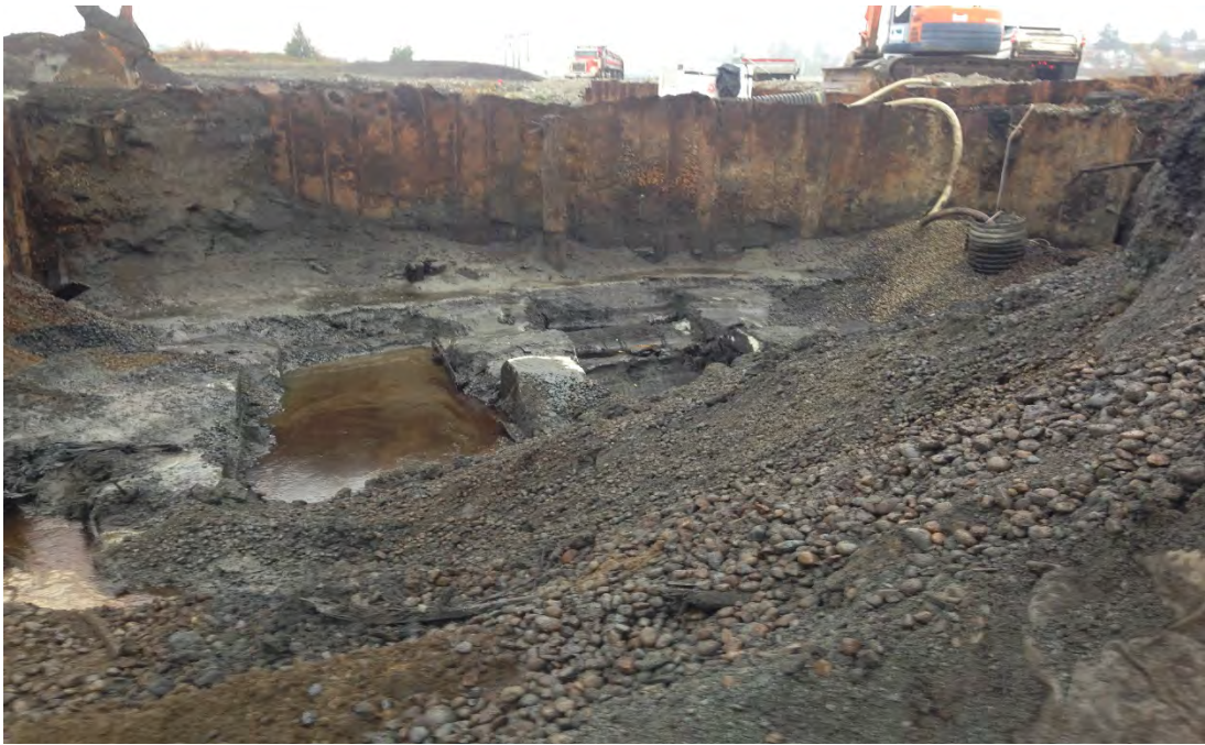
Photograph 29 – USTs 71, 72, 73 excavation: looking east across USTs location to north-south-trending sheet pile wall
