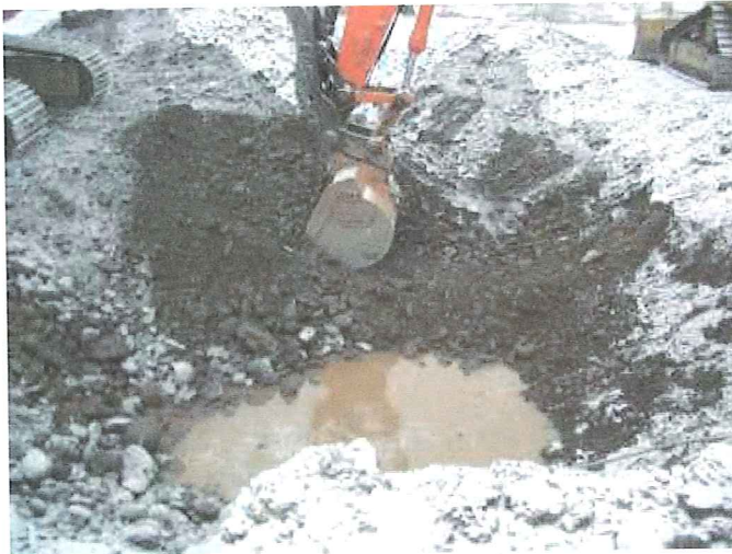
Photo 03 - Water in excavation west end - 6' bgs
