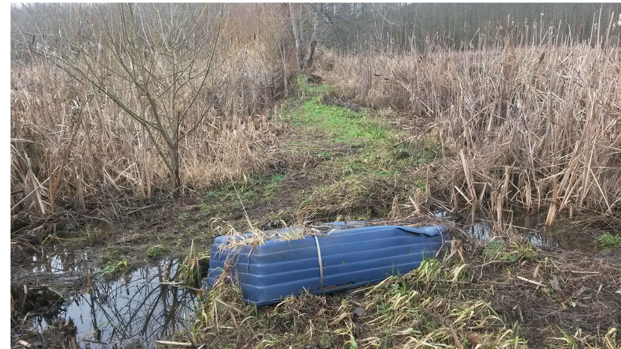
PHOTO B/CG09.1 SOUTH LAKE BERM LOW SPOT
