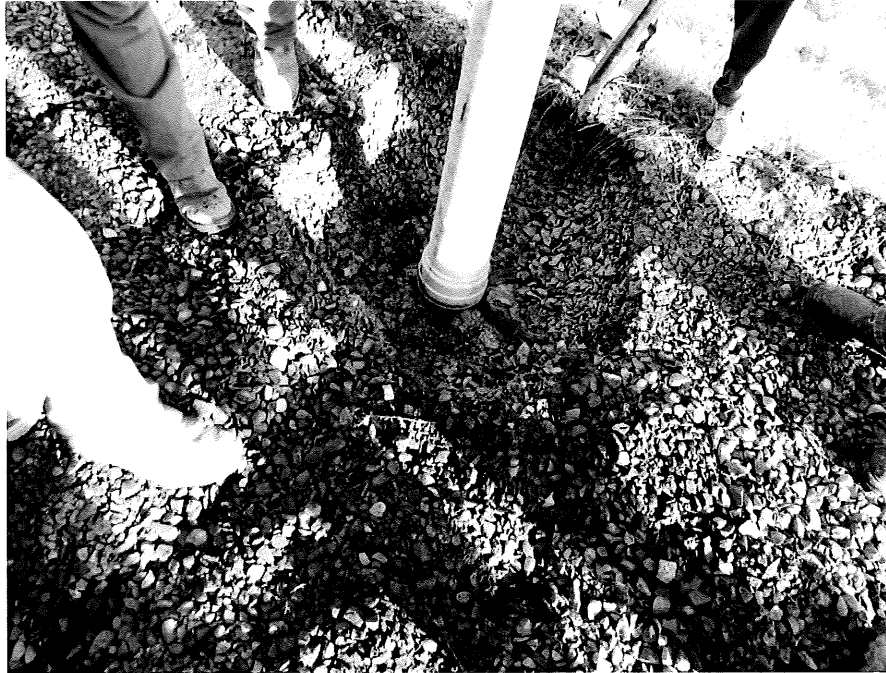
Photograph No. 1: View of the vector truck removing gravel and soil for exposing utilities.
