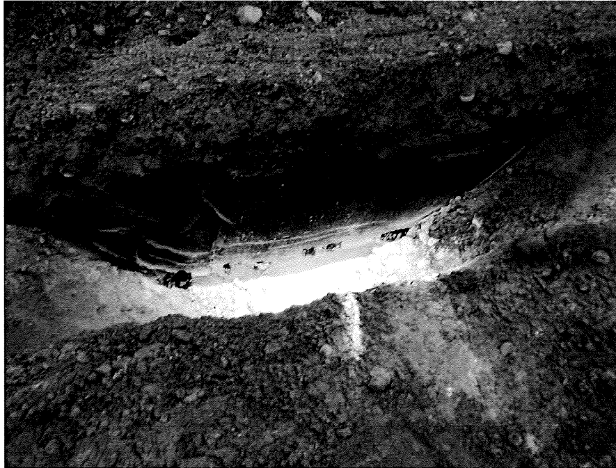
Photograph No. 7: View of the application of the remedial amendment prior to hydrating and mixing. Water is observed seeping in from lower sidewall.
