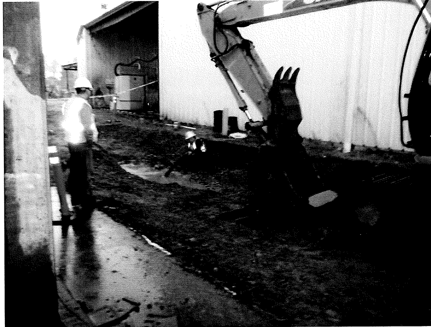
Photograph No. 5: View of the storm water being pumped from the approximate 4 foot excavation on the eastern end of excavation area.
