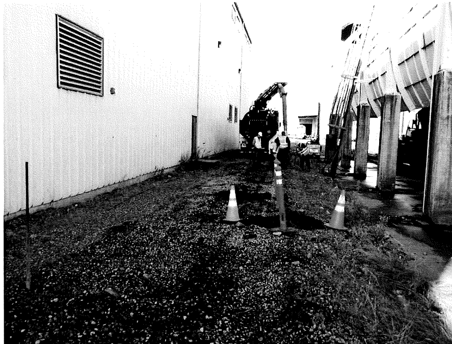
Photograph No. 3: View of the track gravel area with the tracks removed, gradually sloping to the north (wash pad located on right side of photo).
