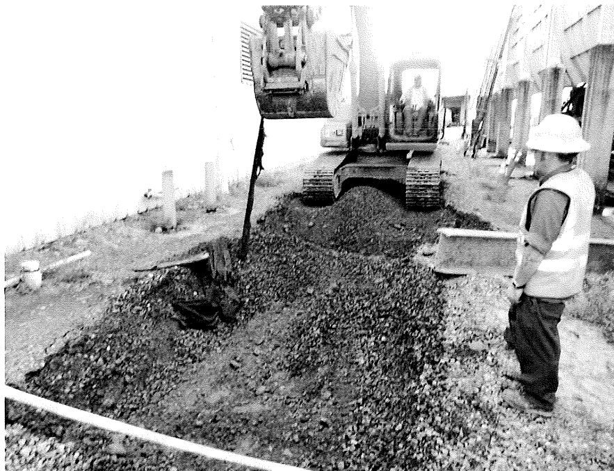
Photograph No. 4: View of the gravel, filter fabric and soils being excavated on the east end of the excavation area.
