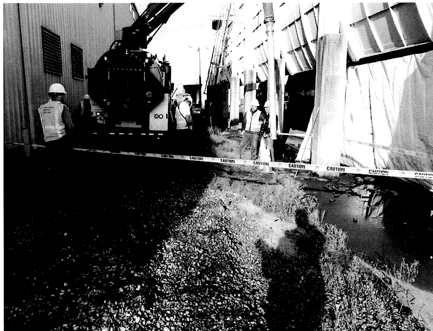
Photograph No. 2: View of NRC completing additional potholes to verify utility locations, facing west.
