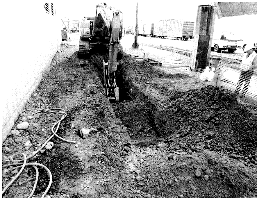
Photograph No. 6: View of the trenching activities for direct application of the remedial amendment.
